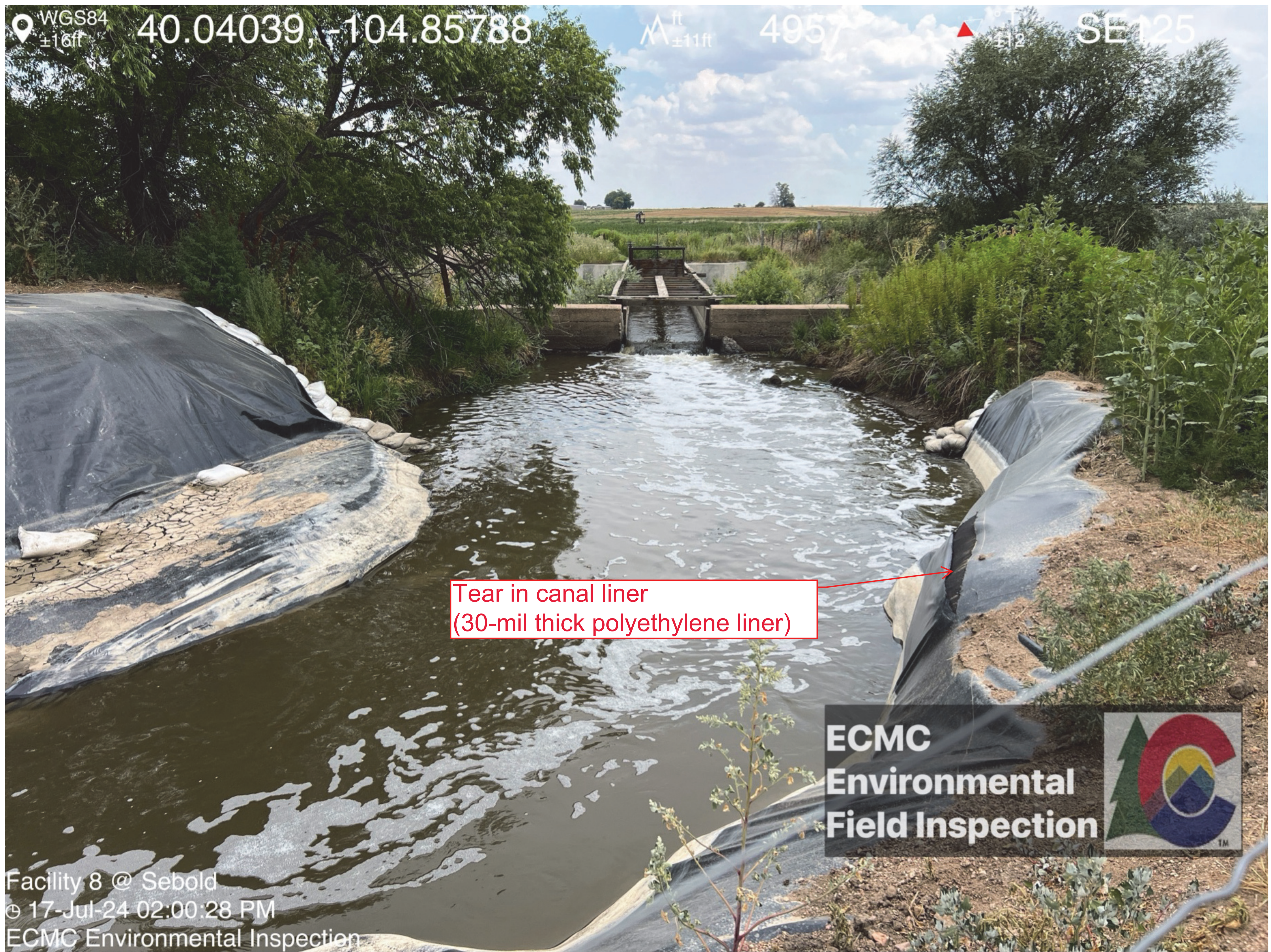
Weeds, tear in 30-mil polyethylene canal liner.
