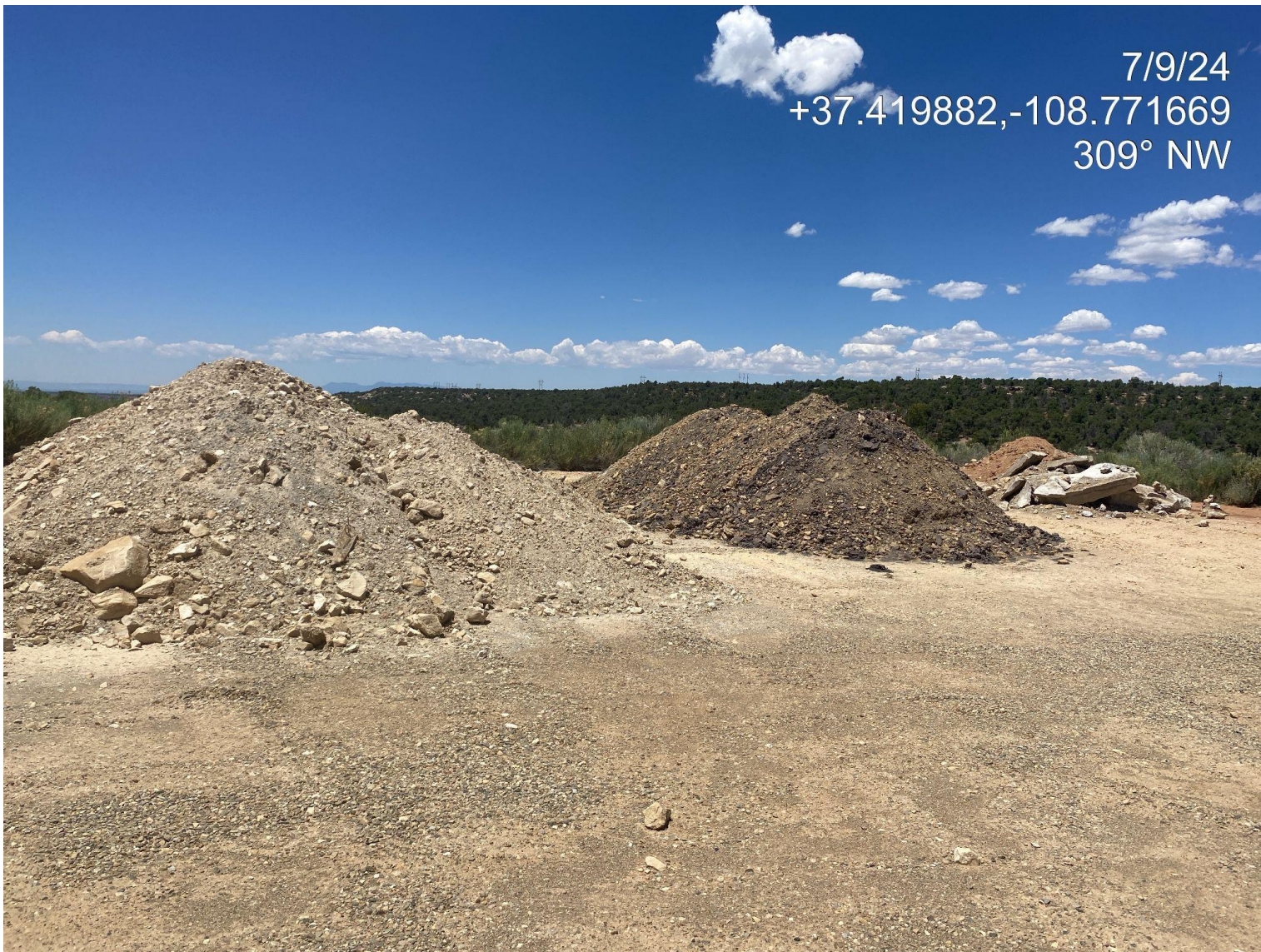
Photo 2. View of removed material from around well head stored on location. Note: if soil is contaminated additional BMPs need to be installed during the storing process.
