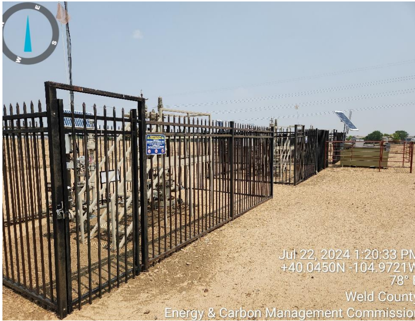
Photo 1 well heads and equipment
