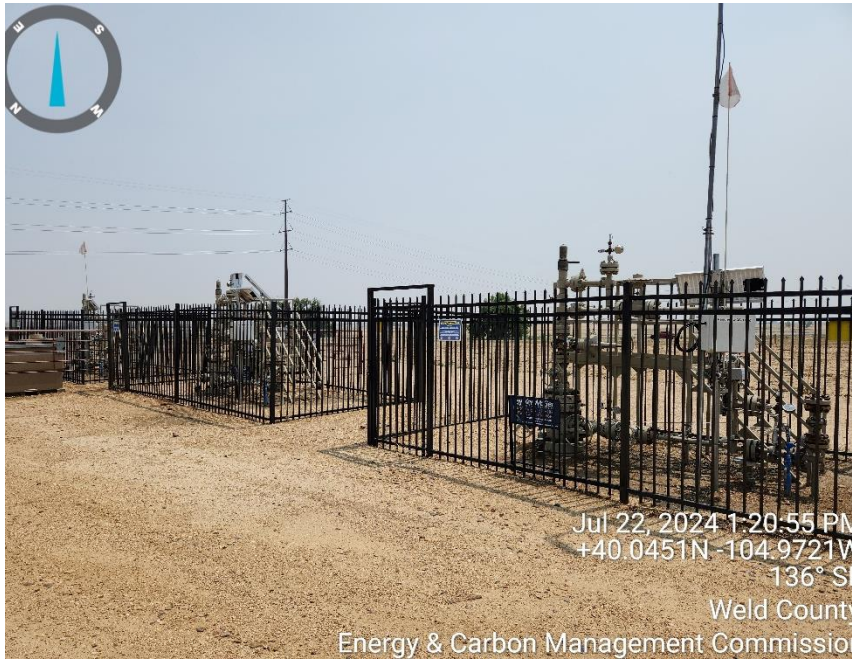
Photo 2 well heads and equipment
