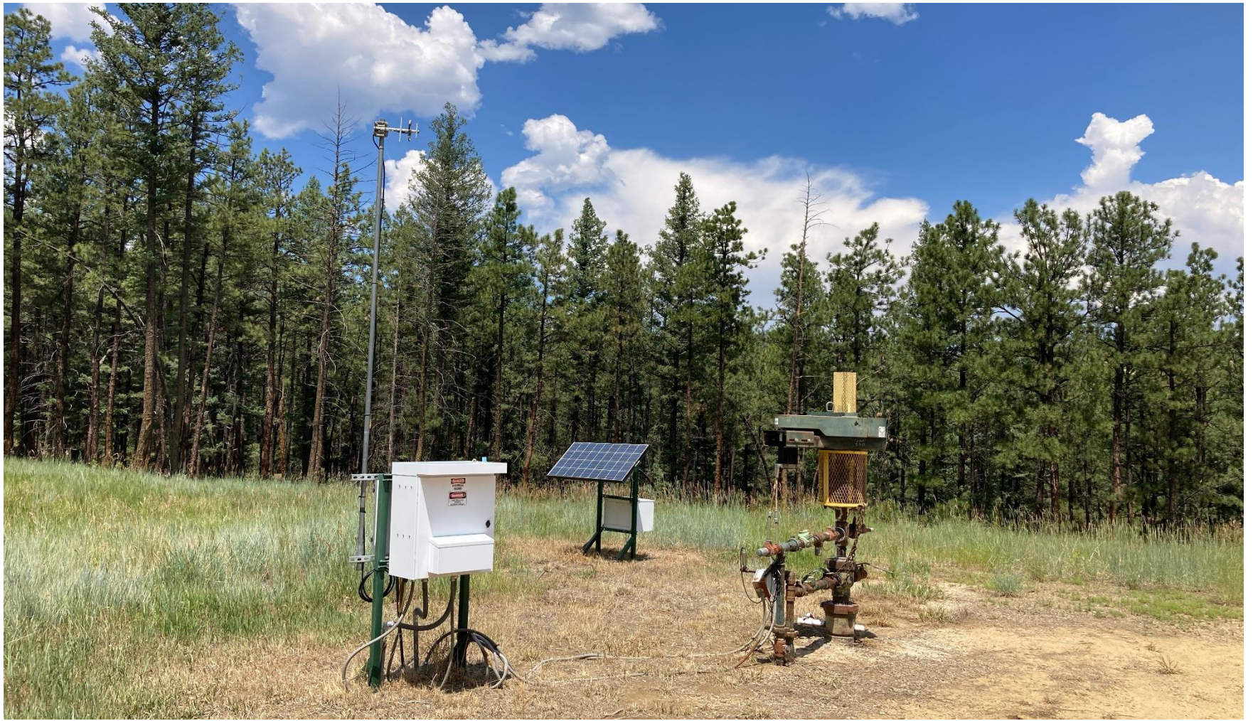
PHOTO 4: TR WELLHEAD AND EQUIPMENT
