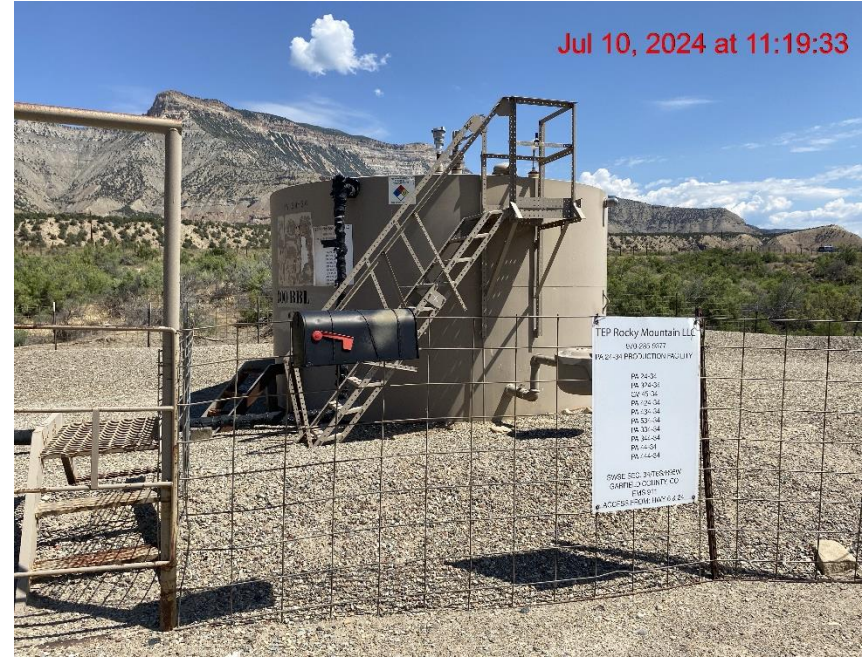
Tank Battery – Photo #02198
