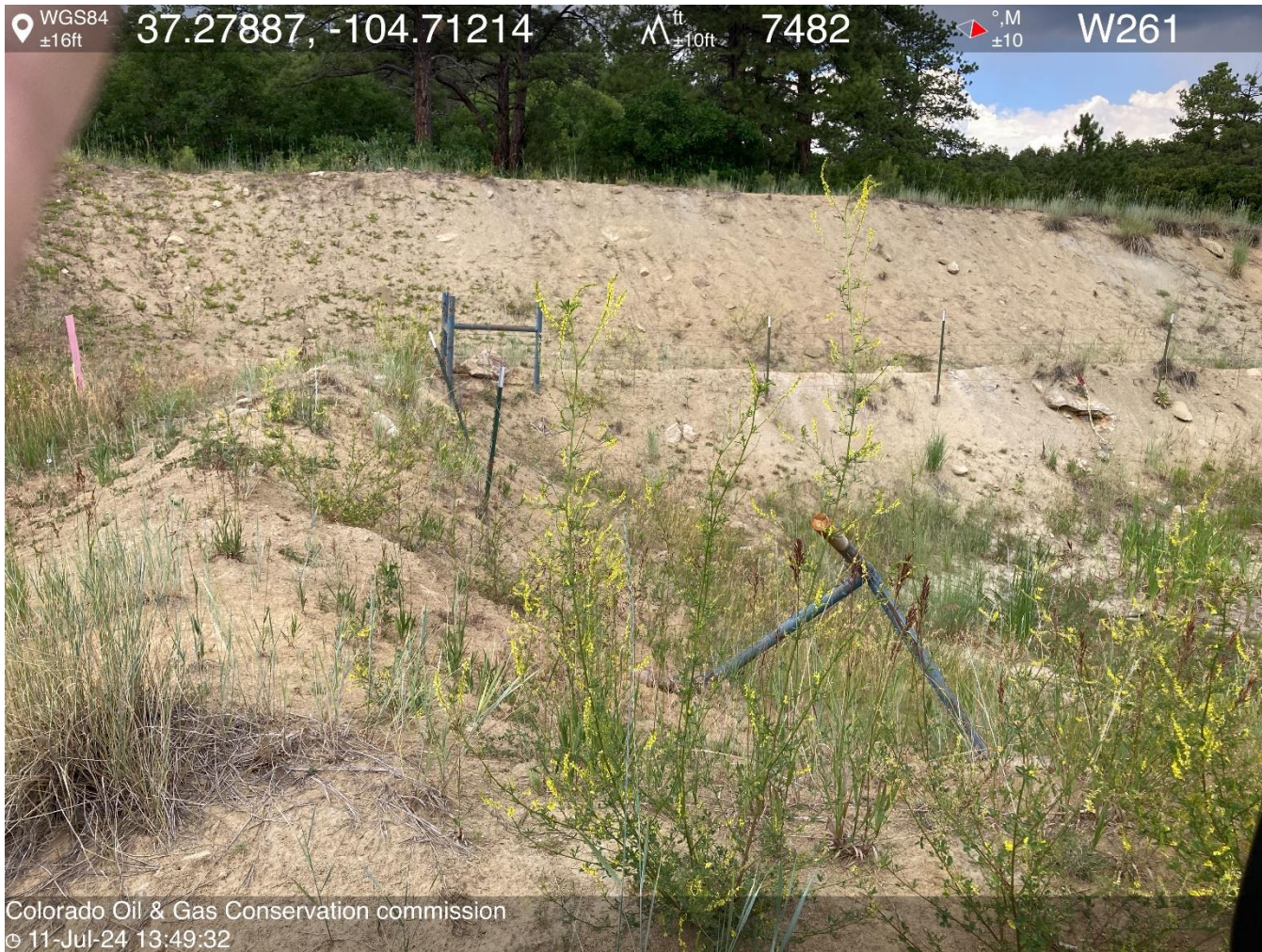
PHOTO 5: FENCE AROUND PIT IS FALLING INTO PIT IN ONE CORNER. REPAIR FENCE PER 1002 RULES.
