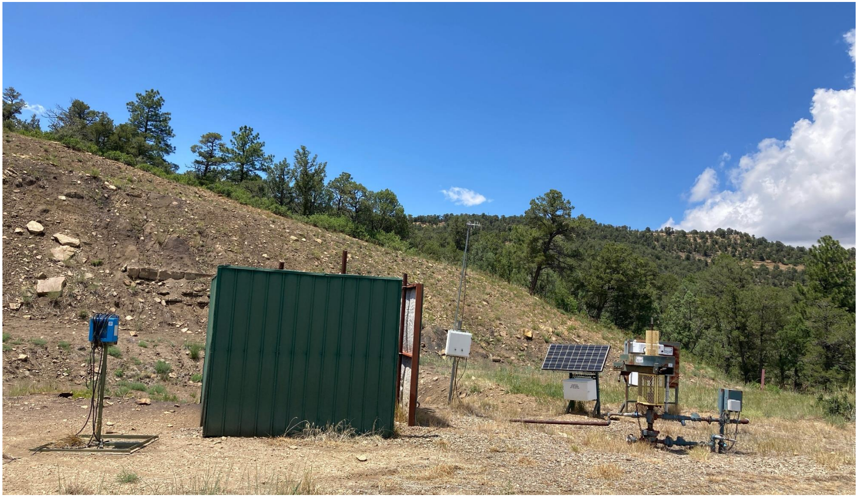
PHOTO 3: WELLHEAD AND EQUIPMENT
