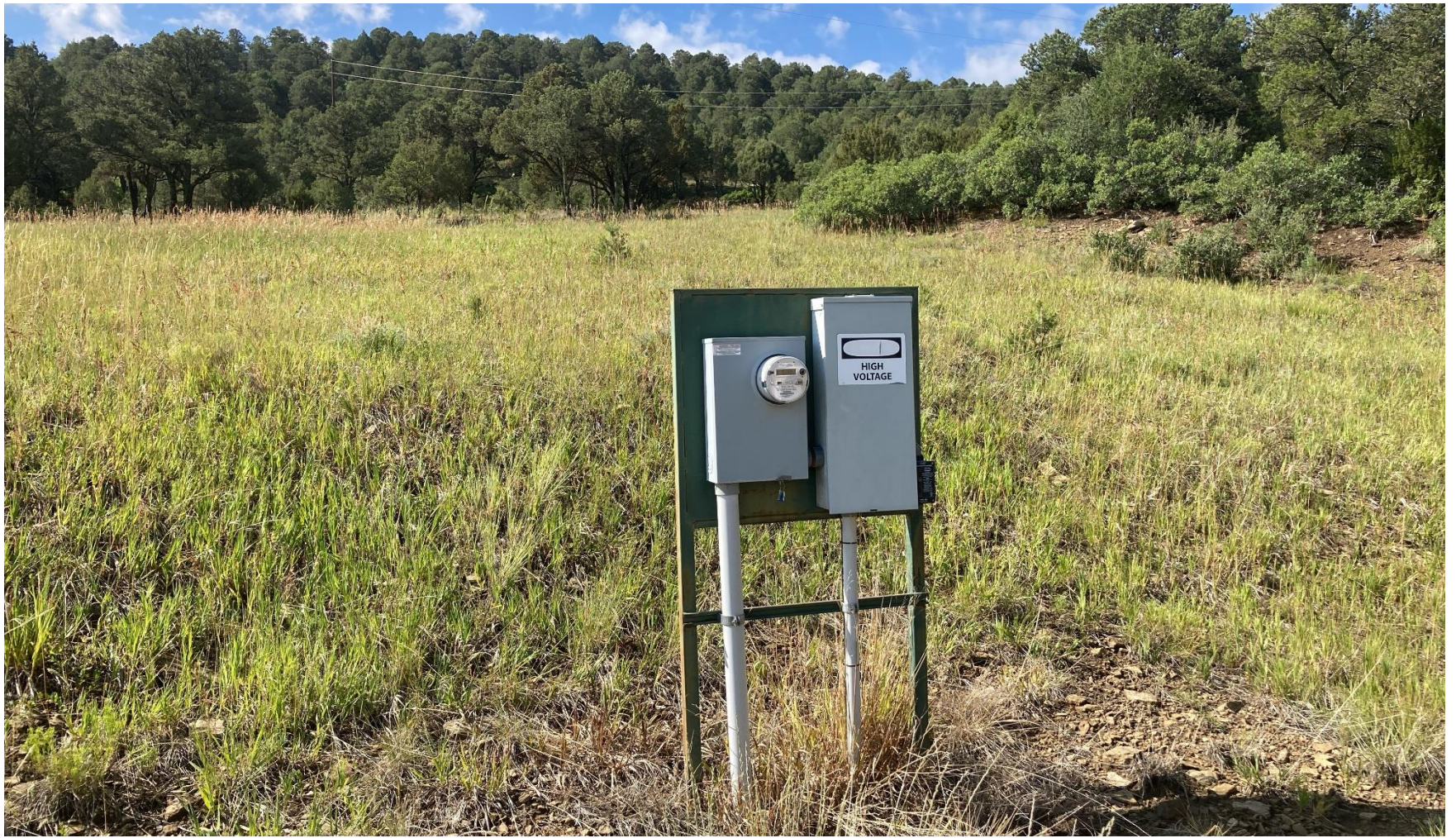
PHOTO 4: ELECTRIC SUPPLY METER.
