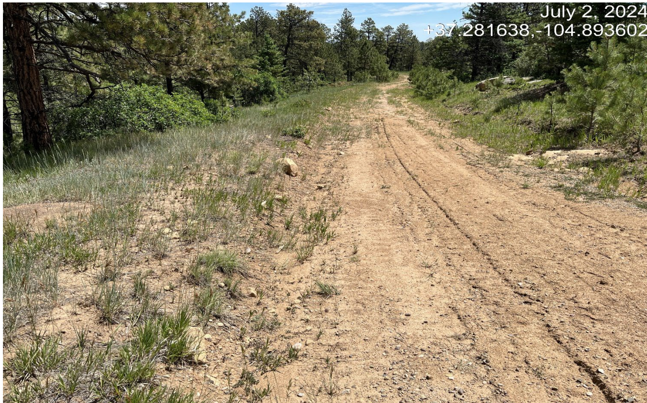
Photo 2. Facing northeast, repairs have been made to areas of the road and BMP's are maintained.
