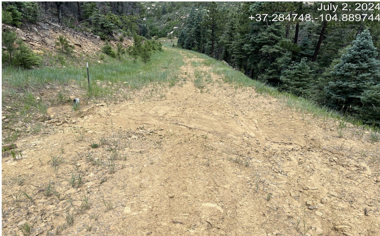
Photo 4. Facing northwest, water bars have been put in to direct stormwater to the culvert.
