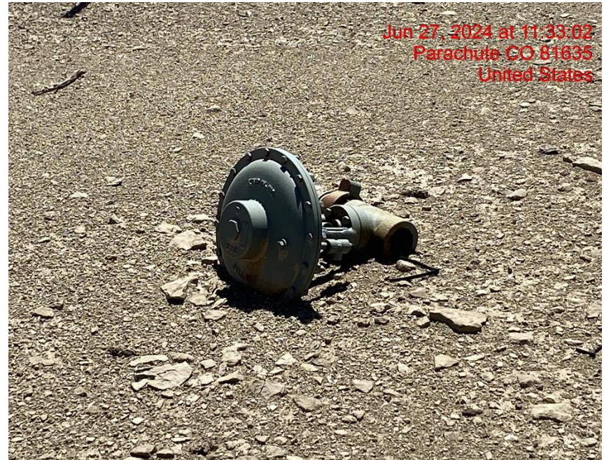
Unused Equipment – Photo #01992
