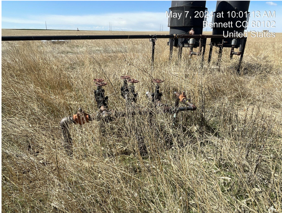
Photo 3. Photo taken facing southwest of pipe risers and burners.
