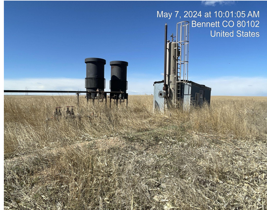
Photo 4. Photo taken facing southwest of burners and separator.
