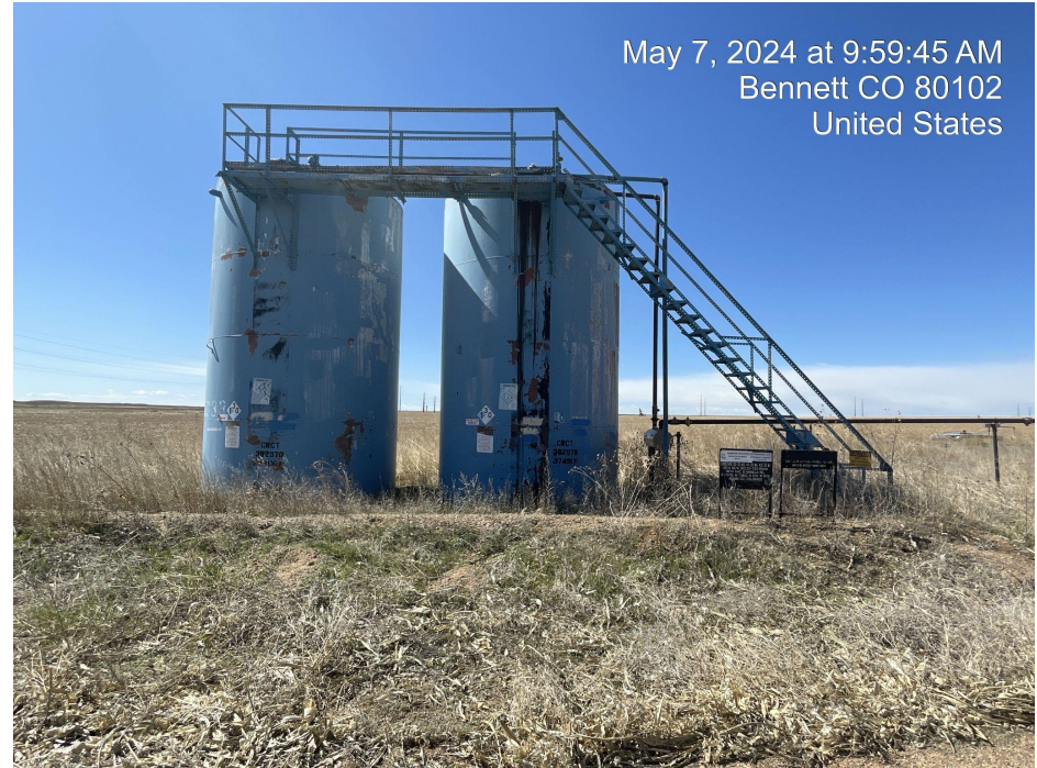
Photo 2. Photo taken facing south of tank battery.
