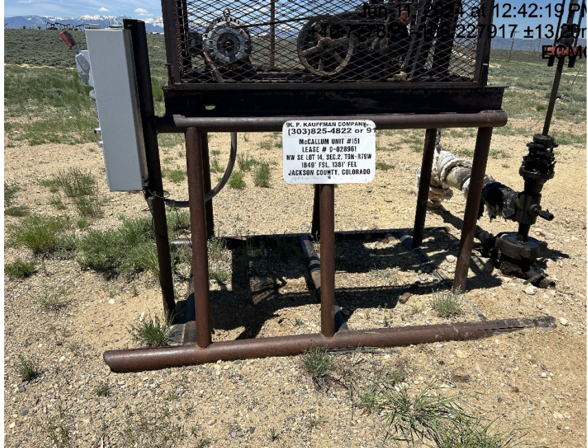
Missing/illegible information on well head signage
