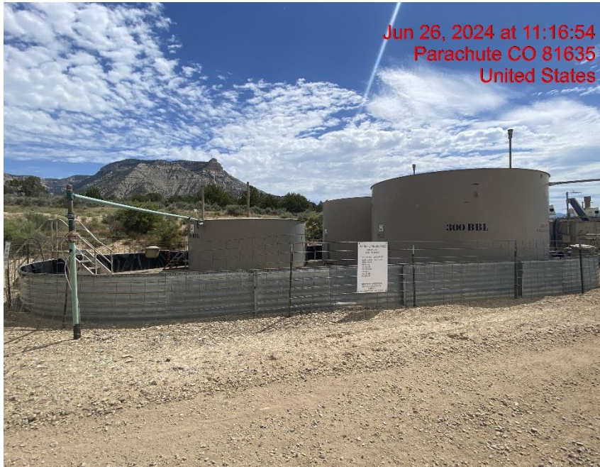
Tank Battery – Photo #01855
