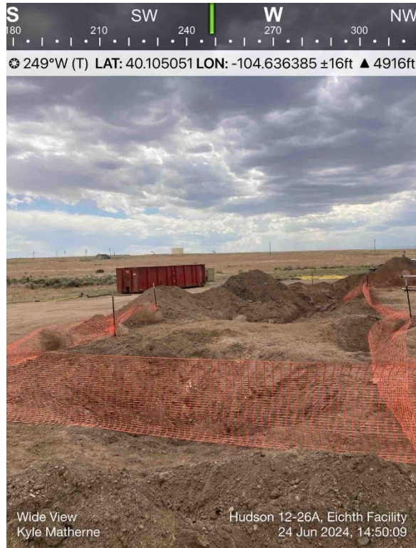
Tank Battery Wide View
