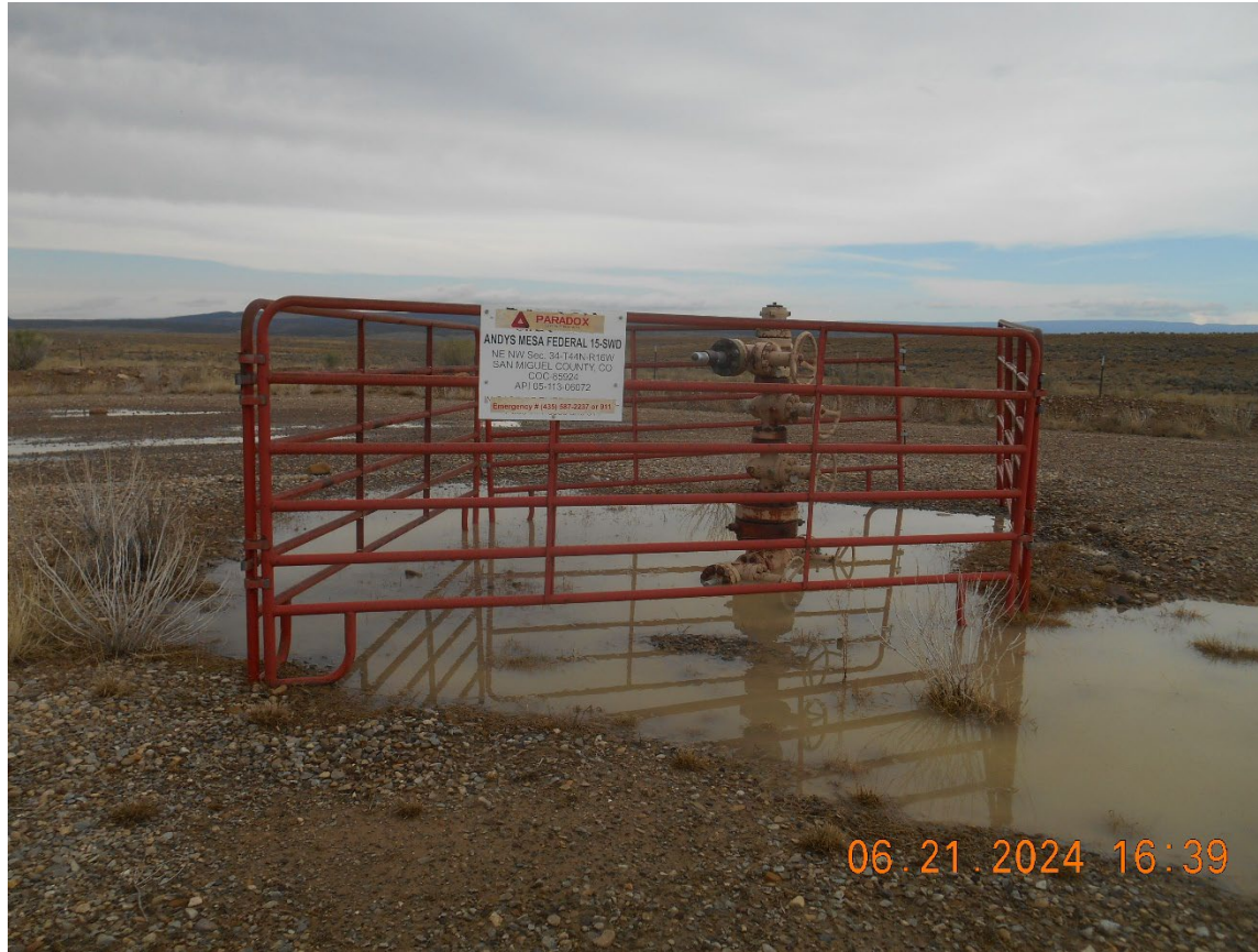
Injection Wellhead. Temporarily abandoned.
