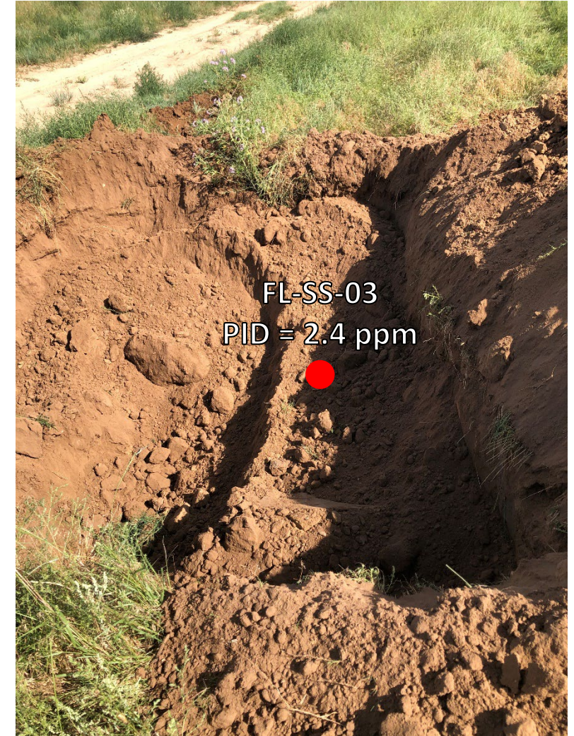
Looking north at cut point for abandonment to Pt B – sample submitted for analysis
