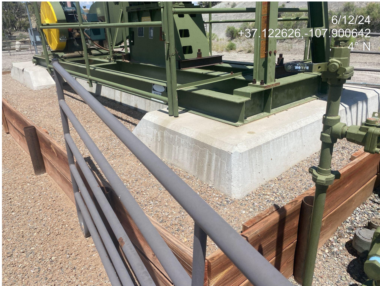
Photo 4. Unused oil and gas equipment corrective action identified in the previous inspection doc #714000499 has been addressed/resolved.
