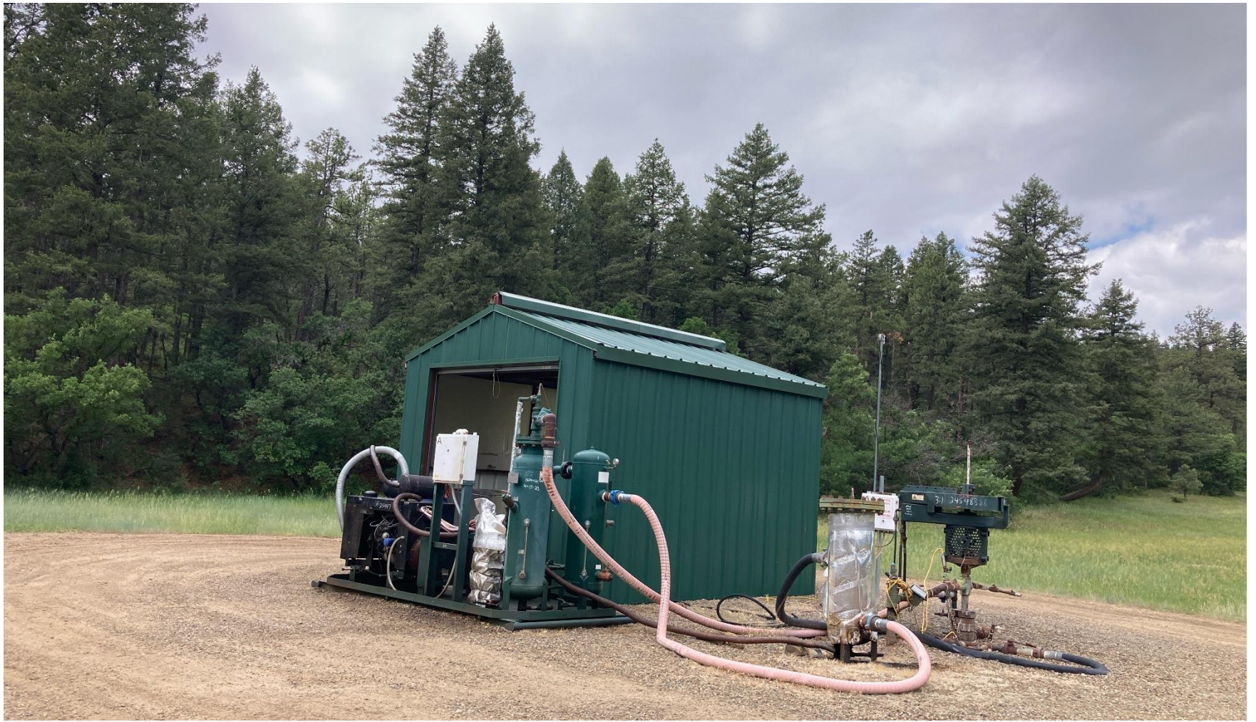
PHOTO 3: WELLHEAD AND EQUIPMENT
