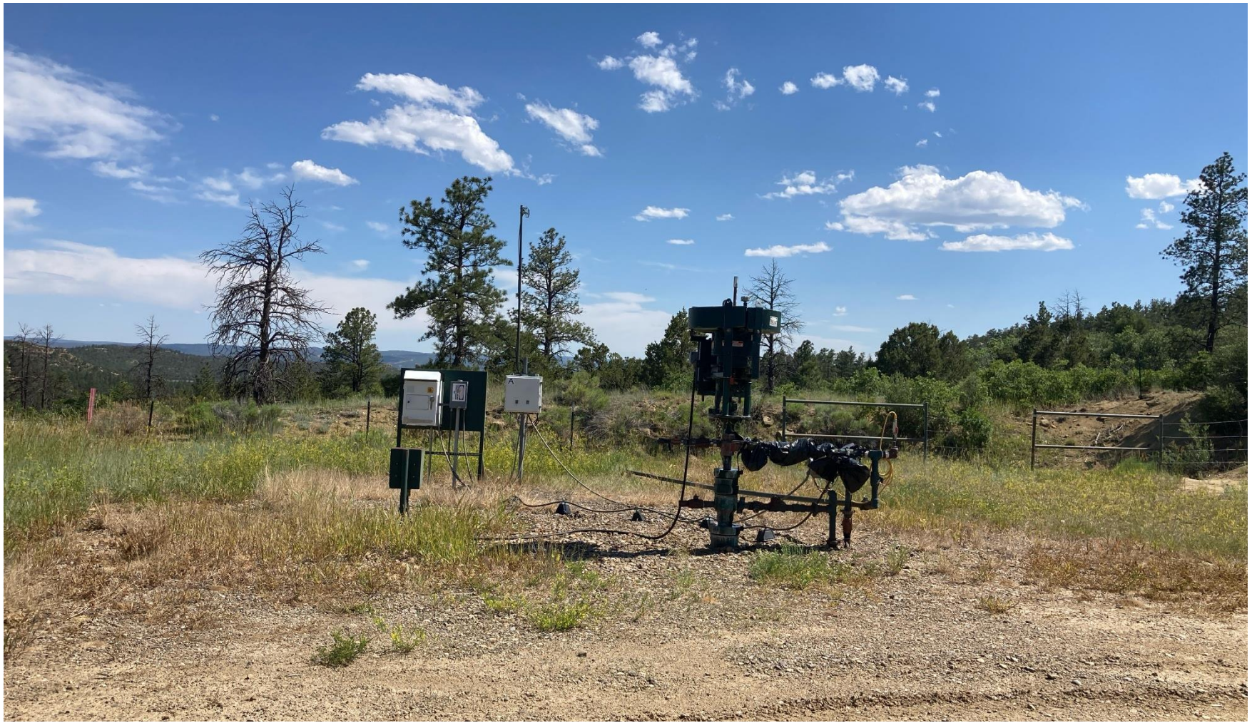
PHOTO 3: WELLHEAD AND EQUIPMENT
