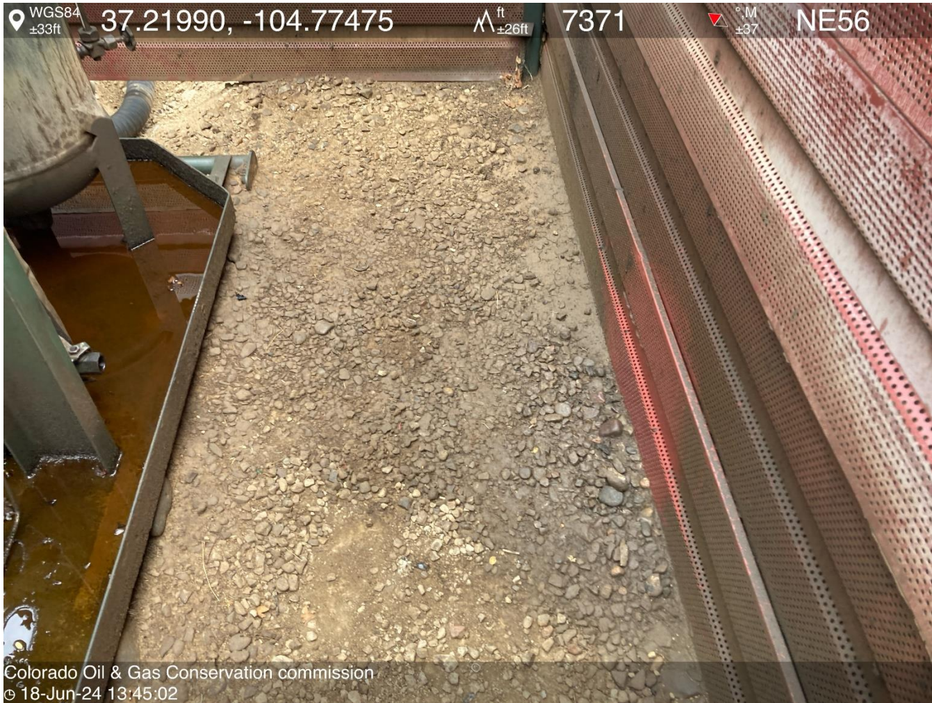
PHOTO 5: STAINED SOIL NEAR COMPRESSOR SKID (SPOKE WITH ZEKE SANCHES TO HAVE THIS CLEANED UP).
