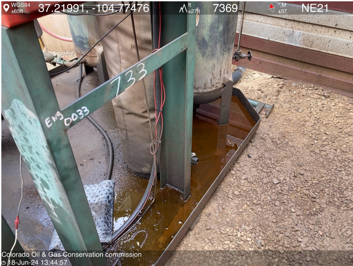
PHOTO 4: OIL IN COMPRESSOR SKID (SPOKE WITH ZEKE SANCHES TO HAVE THIS CLEANED UP).
