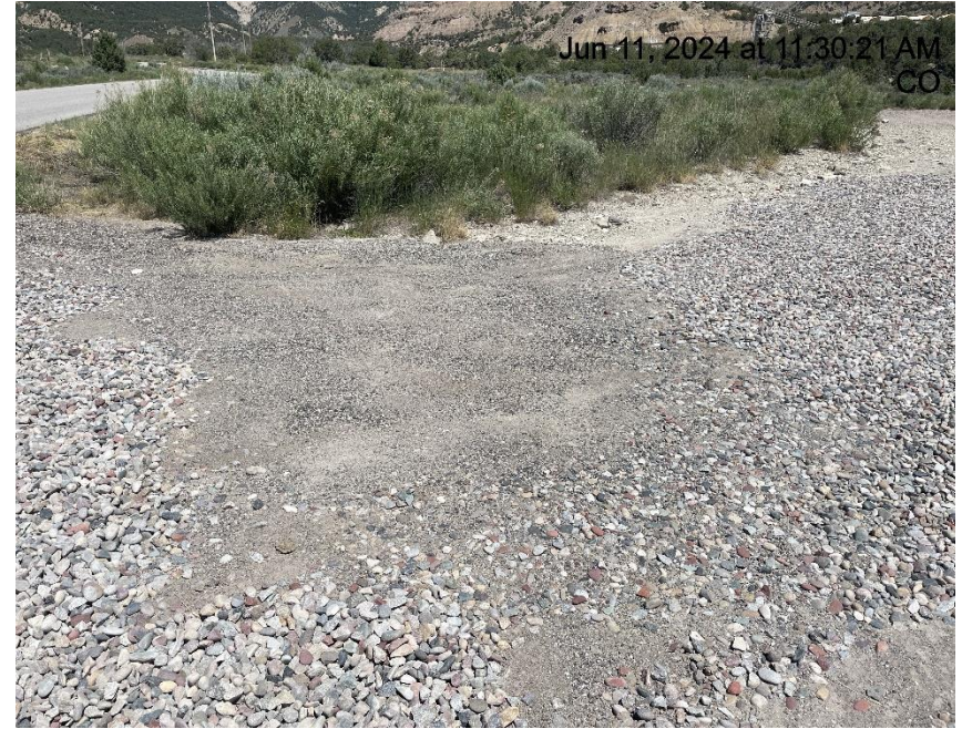
Photo # 444 Sediment migrating onto gravel track pad/BMP needs maintenance
