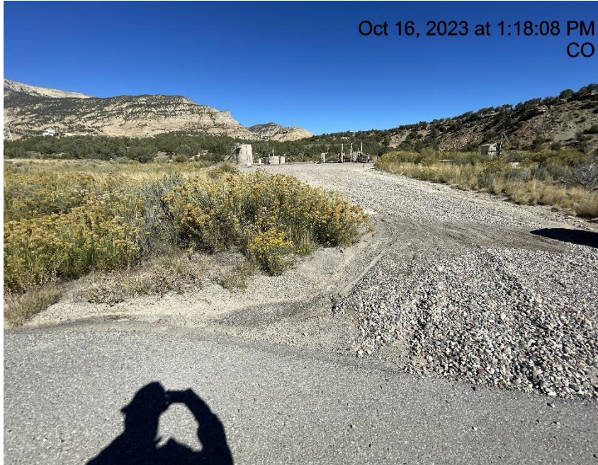
Photo # 2885 From inspection 708901973 conducted on 10/16/2023 Sediment migrating onto gravel track pad/BMP needs maintenance
