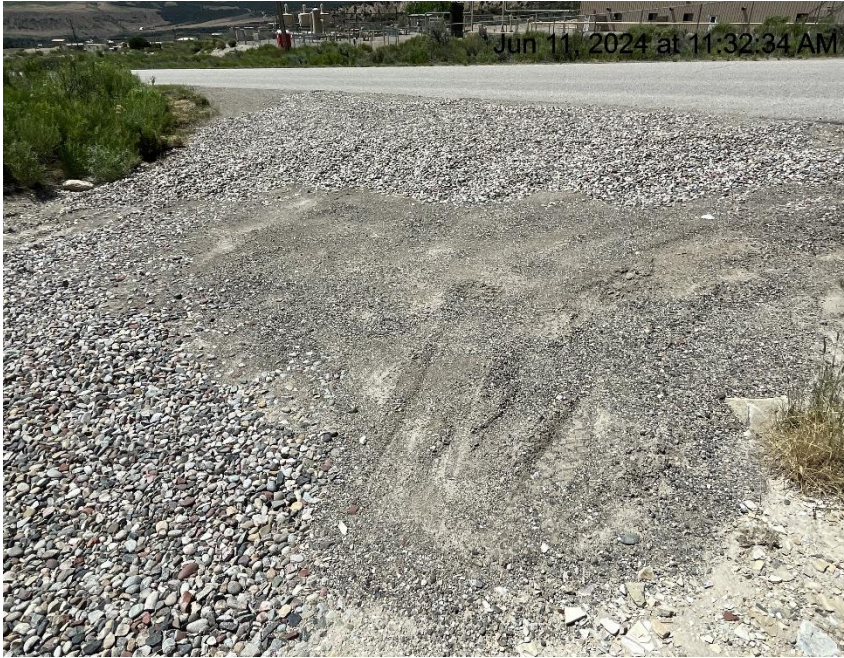
Photo # 443 Sediment migrating onto gravel track pad/BMP needs maintenance
