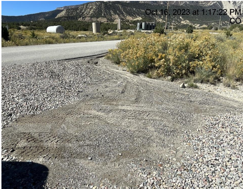
Photo # 2891 From inspection 708901973 conducted on 10/16/2023 Sediment migrating onto gravel track pad/BMP needs maintenance
