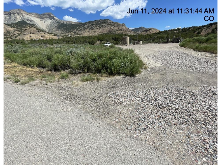
Photo # 436 Sediment migrating onto gravel track pad/BMP needs maintenance
