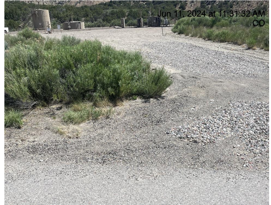
Photo # 435 Sediment migrating onto gravel track pad/BMP needs maintenance
