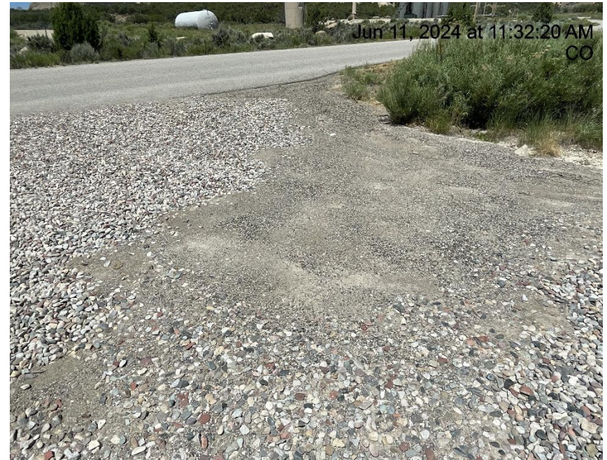
Photo # 441 Sediment migrating onto gravel track pad/BMP needs maintenance
