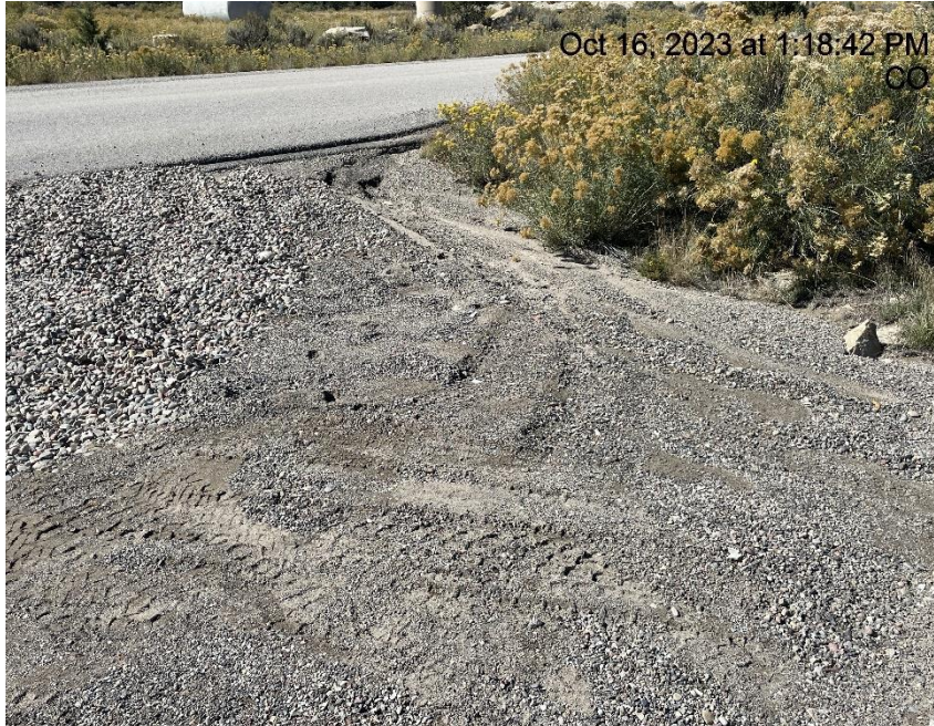
Photo # 2890 From inspection 708901973 conducted on 10/16/2023 Sediment migrating onto gravel track pad/BMP needs maintenance
