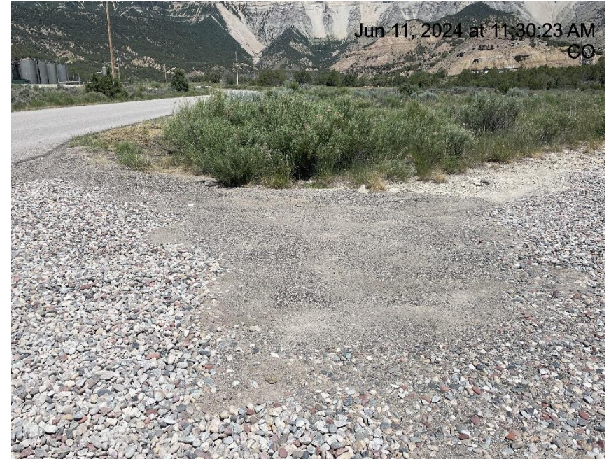
Photo # 440 Sediment migrating onto gravel track pad/BMP needs maintenance
