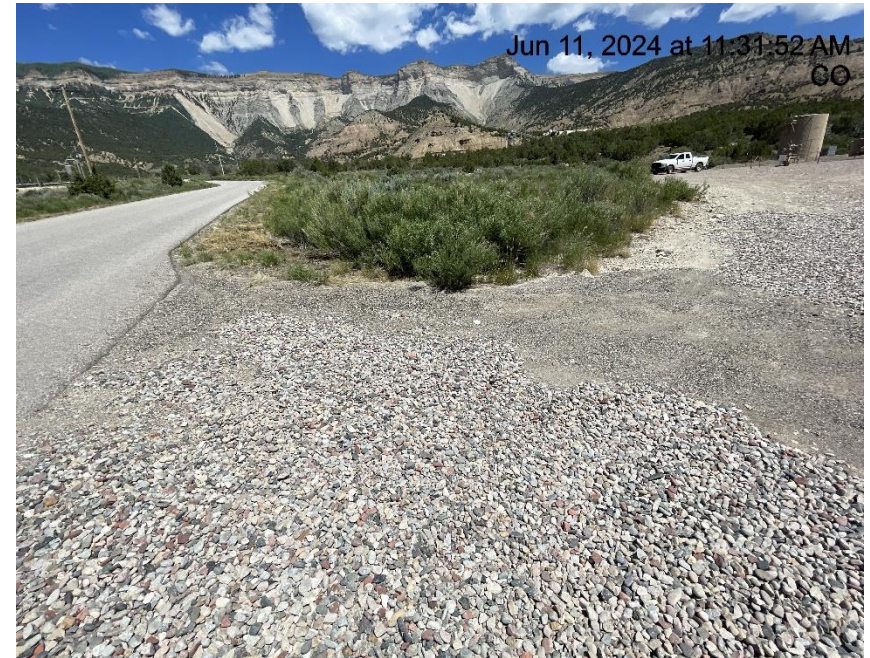
Photo # 437 Sediment migrating onto gravel track pad/BMP needs maintenance
