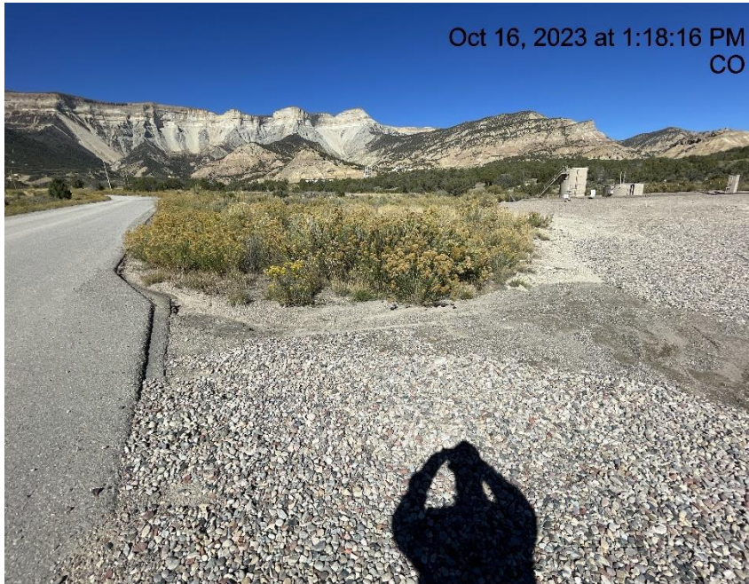
Photo # 2886 From inspection 708901973 conducted on 10/16/2023 Sediment migrating onto gravel track pad/BMP needs maintenance
