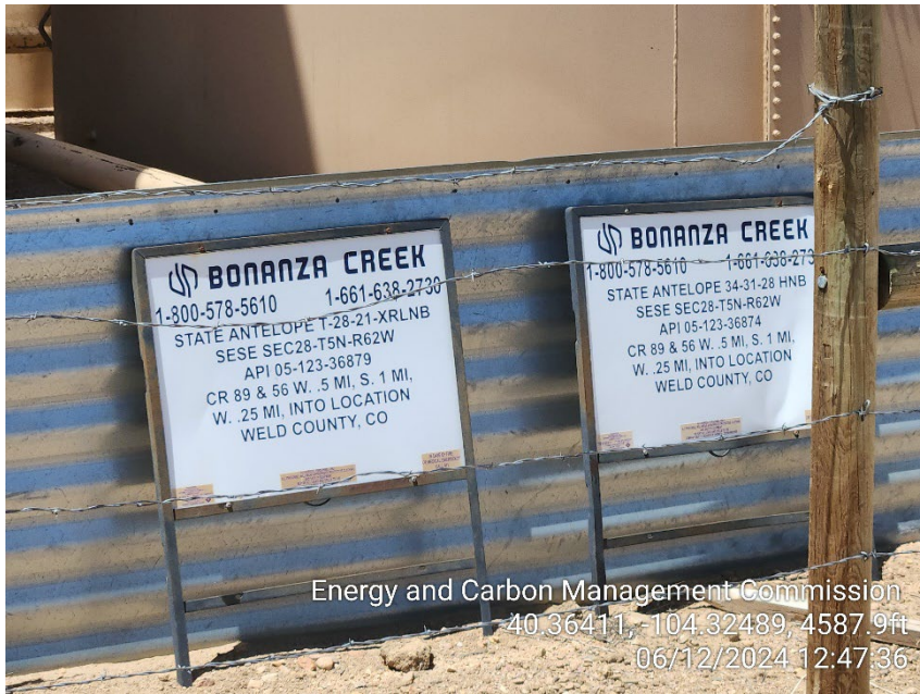
Photo 5 – Gas Lift Injection Meters
