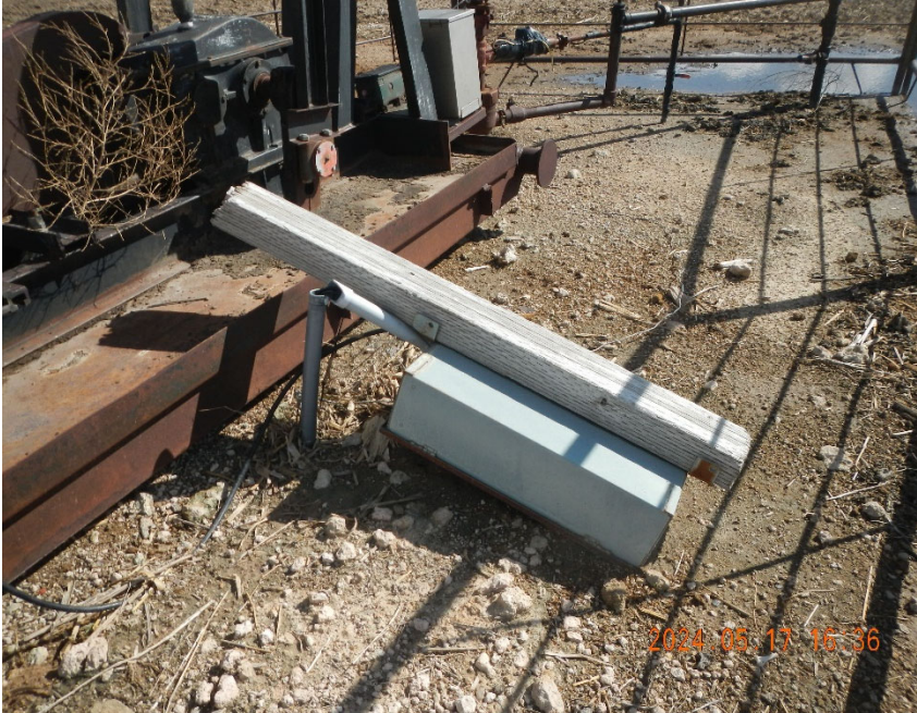
3. Pumping units power and control panel on ground.
