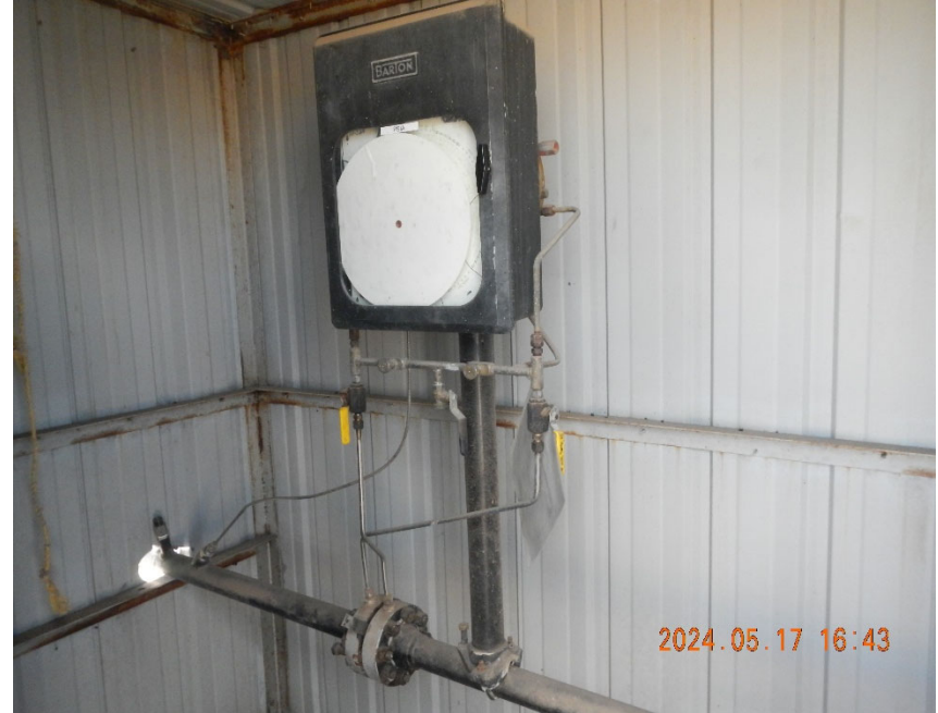
6. Gas meter inside meter shed.
