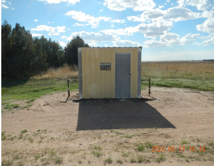
5. Remote gas meter shed.
