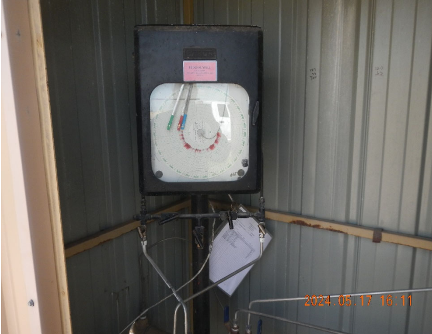
5. Gas meter inside meter shed.
