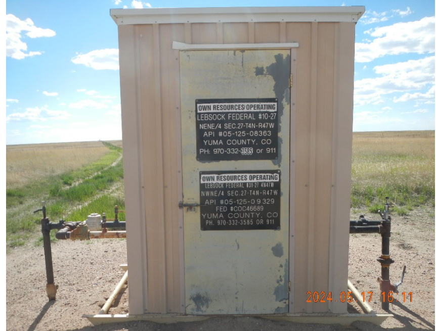
4. Shared remote gas meter shed.
