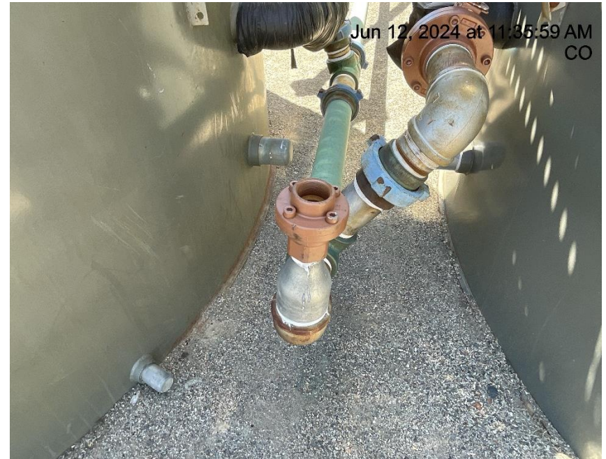
Photo # 569 Open ended load line
