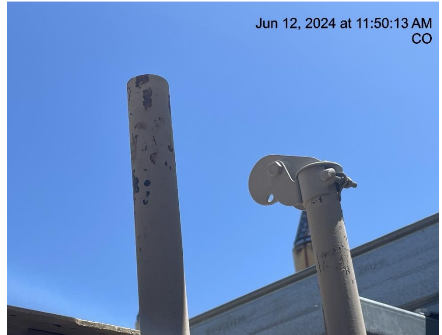
Photo # 553 Rupture disc vent line does not comply with CECMC pressure safety device rules (RWF 533-30 separator)
