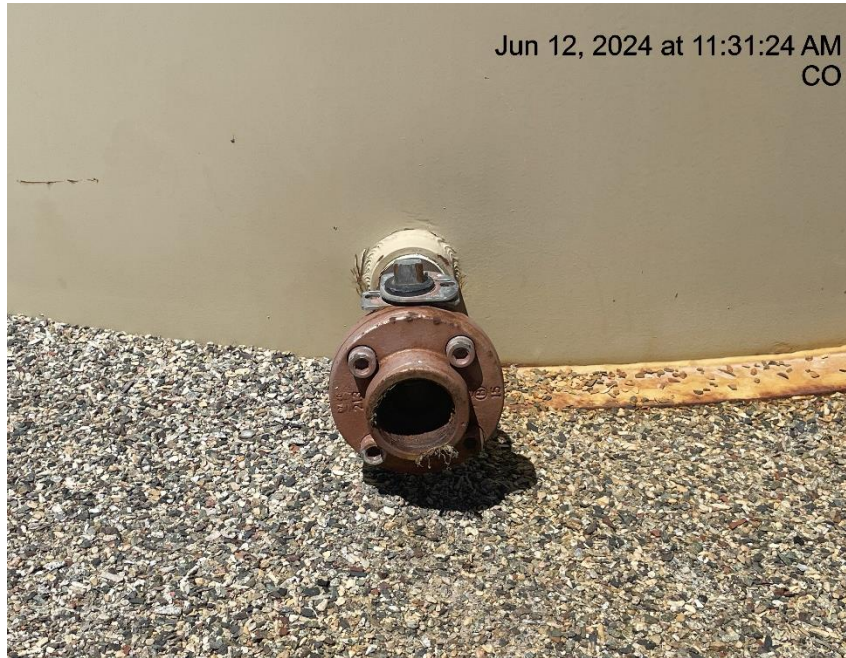
Photo # 566 Open ended load line
