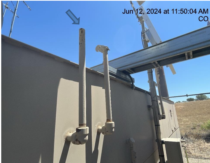
Photo # 552 Rupture disc vent line does not comply with CECMC pressure safety device rules (RWF 533-30 separator)
