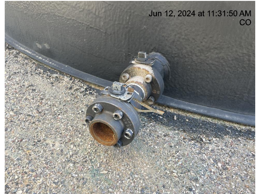
Photo # 567 Open ended load line
