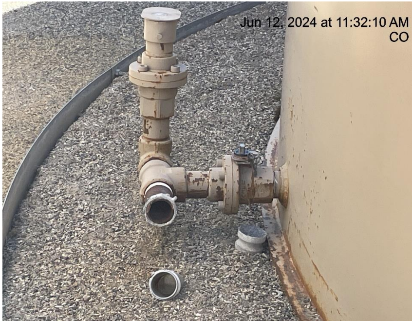
Photo # 568 Open ended load line
