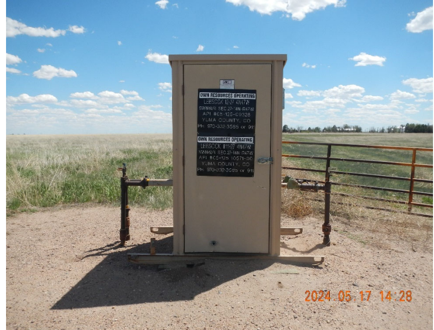
4. Shared remote meter shed.
