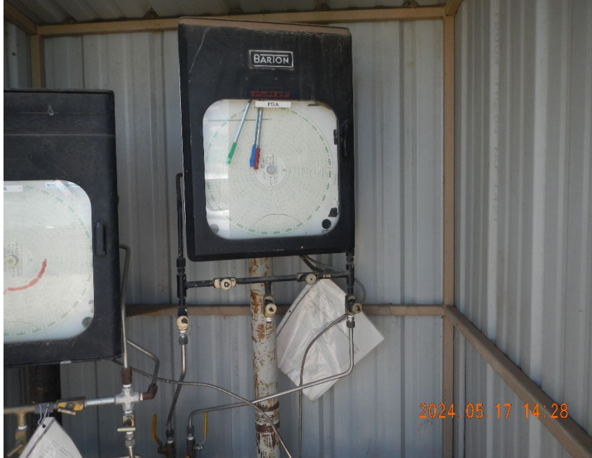
5. Gas meter inside meter shed.
