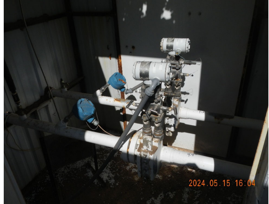
6. Digital gas meter inside meter shed.
