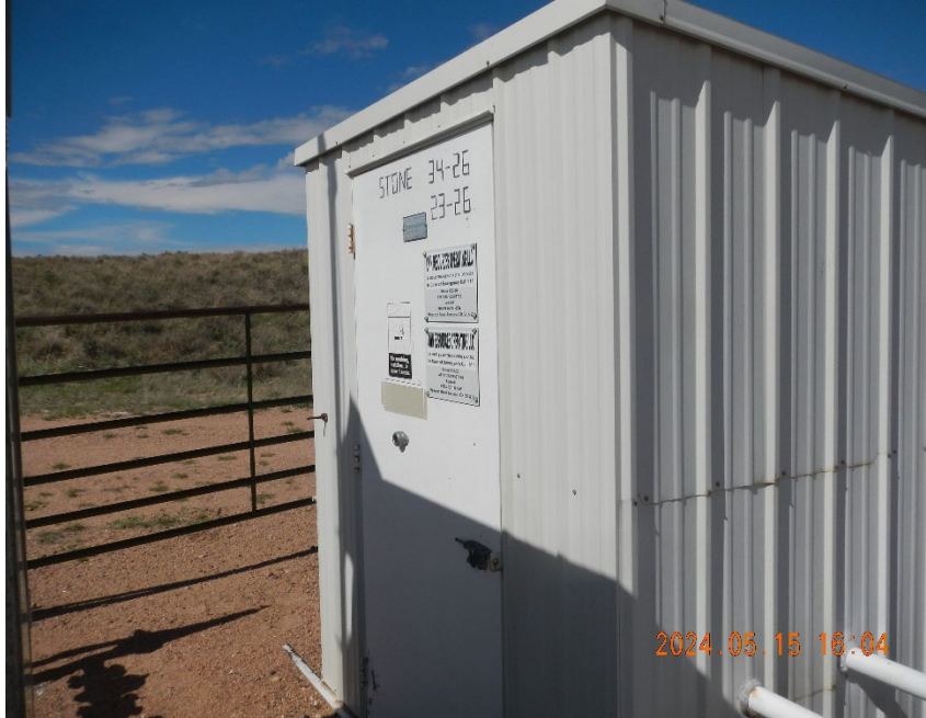
5. Lease signs on shared remote gas meter shed.
