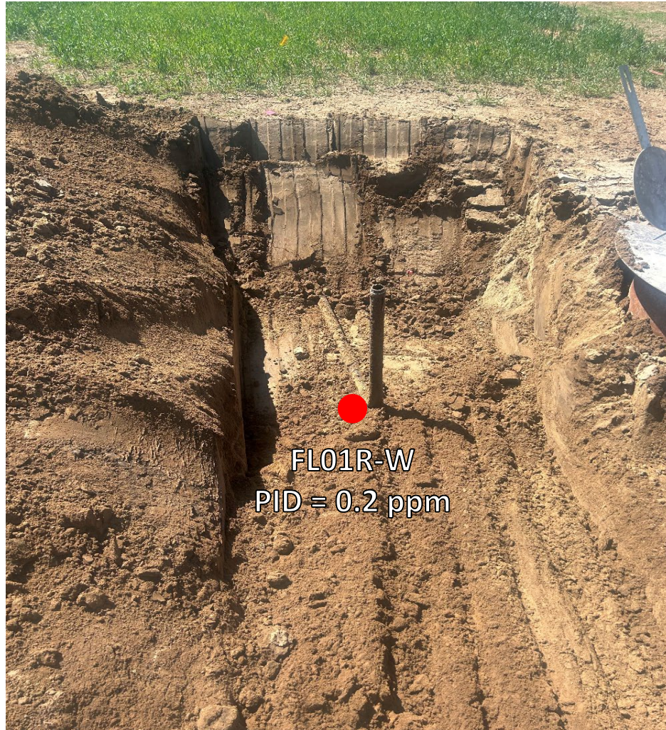
Looking south at flowline Pt A at wellhead
