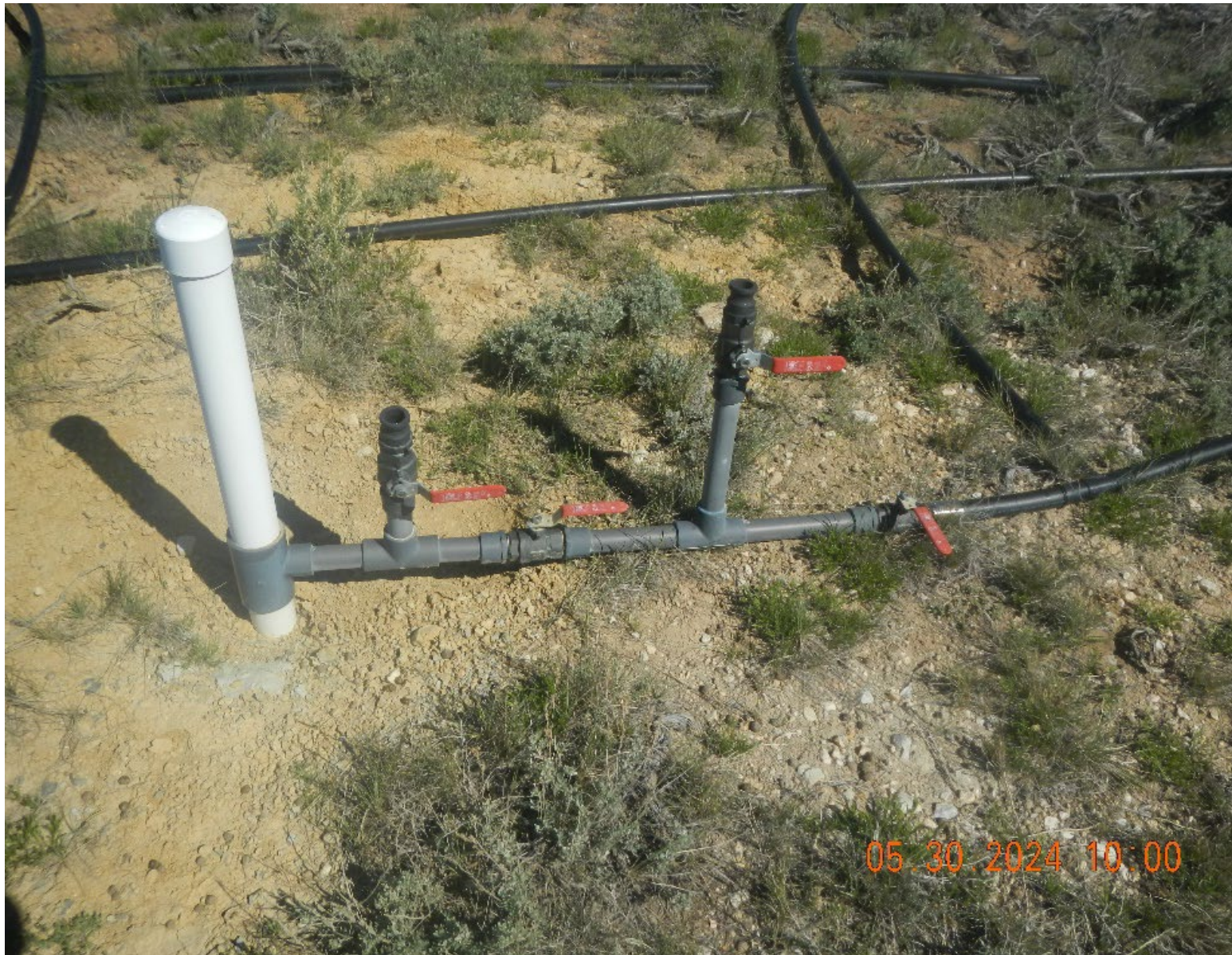
Photo #19 Sparge well and pipe. Note: the position of valve on right, it is throttled.
