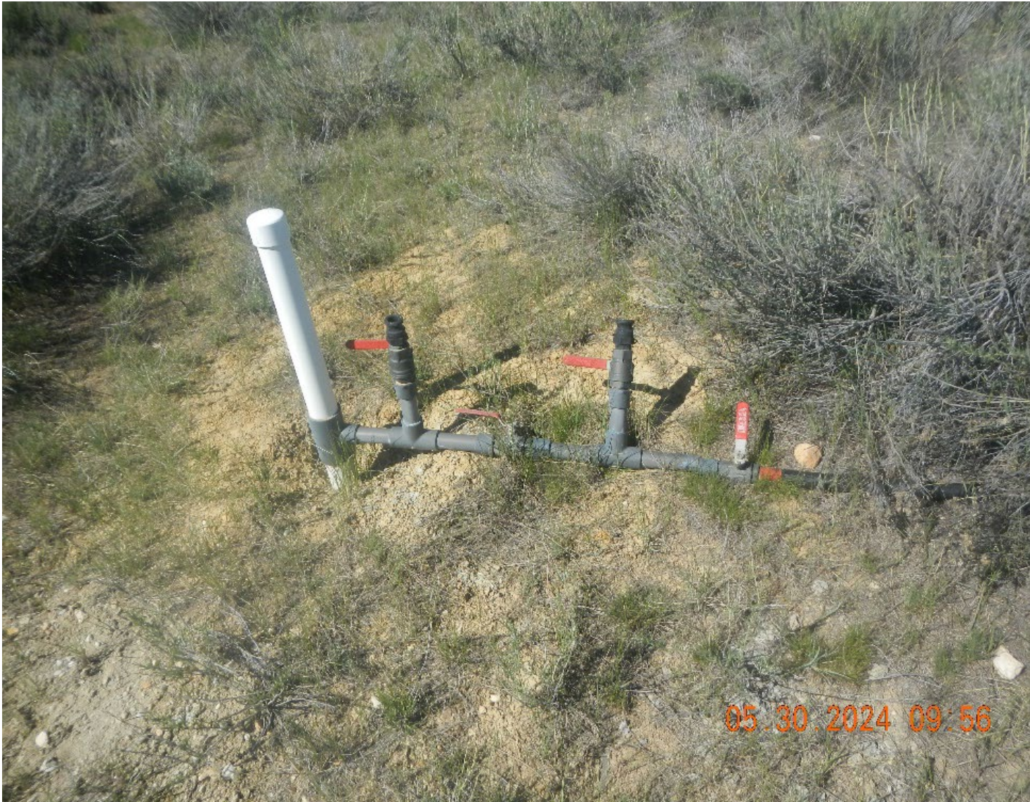
Photo #9 Sparge well and pipe. Note: the position of valve on right, it is closed.
