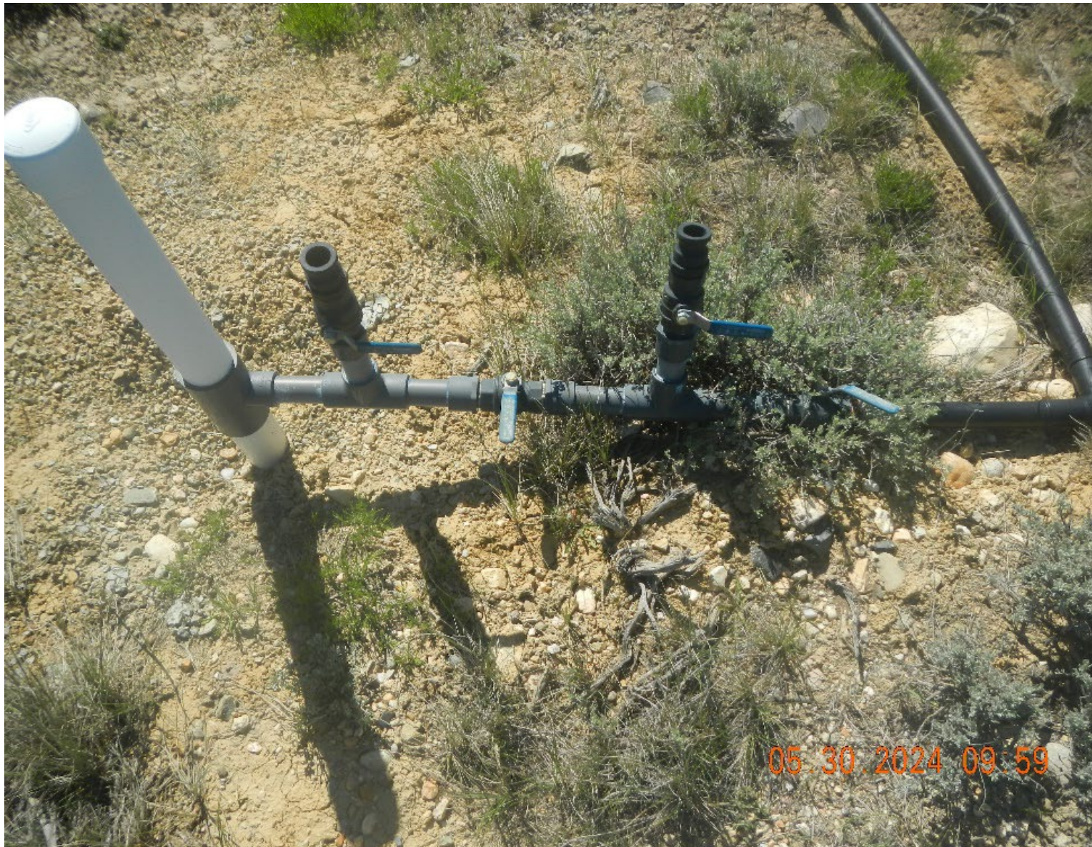
Photo #17 Sparge well and pipe. Note: the position of valve on right, it is throttled.
