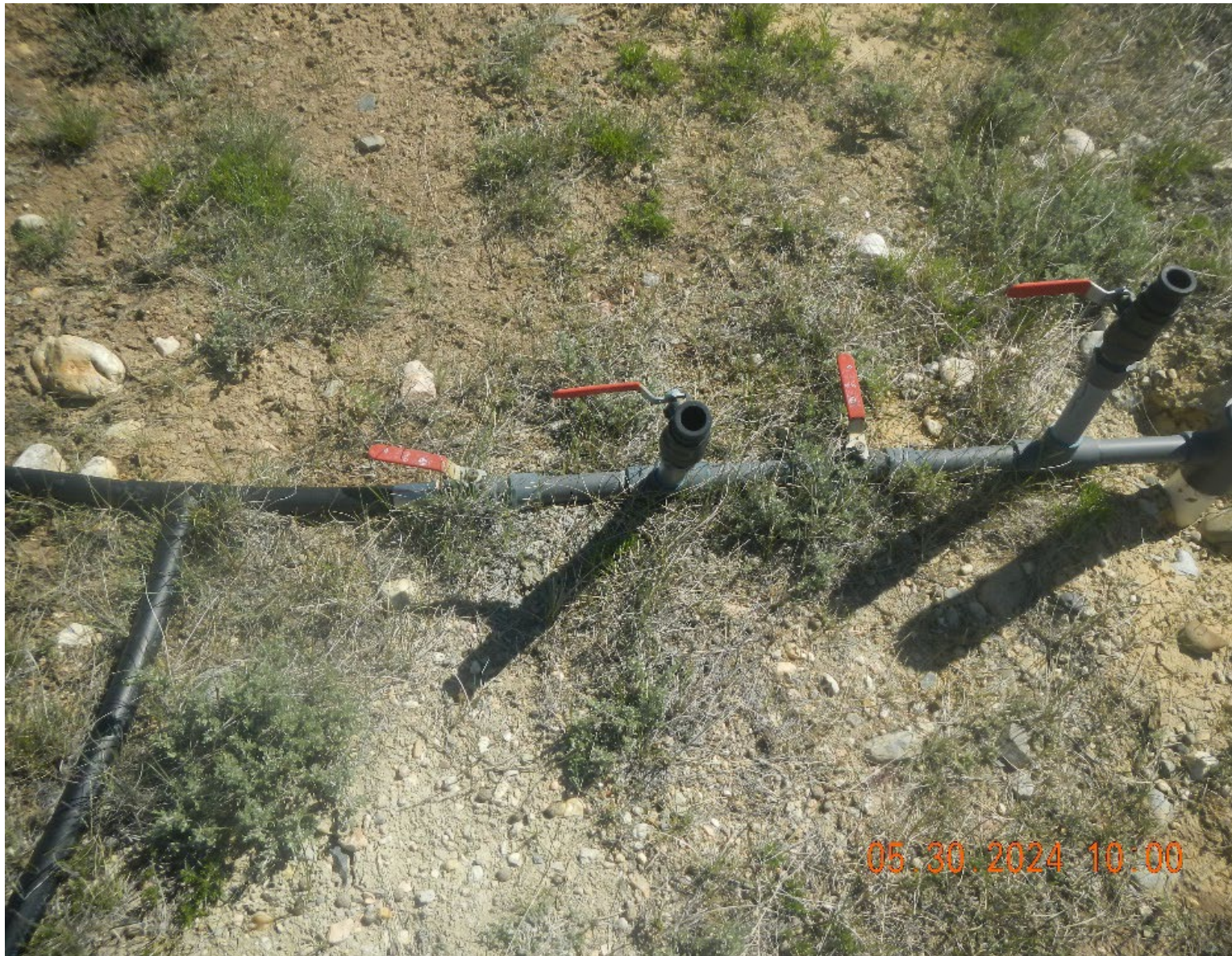
Photo #18 Sparge well and pipe. Note: the position of valves.
