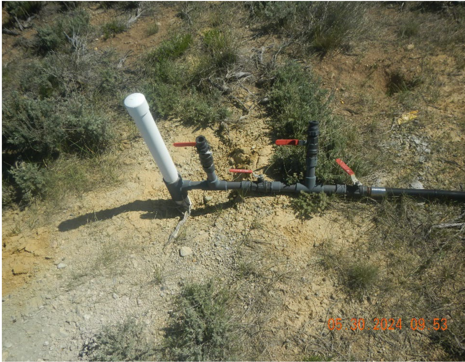
Photo #5 Sparge well and pipe. Note: the position of valve on right, it is throttled.
