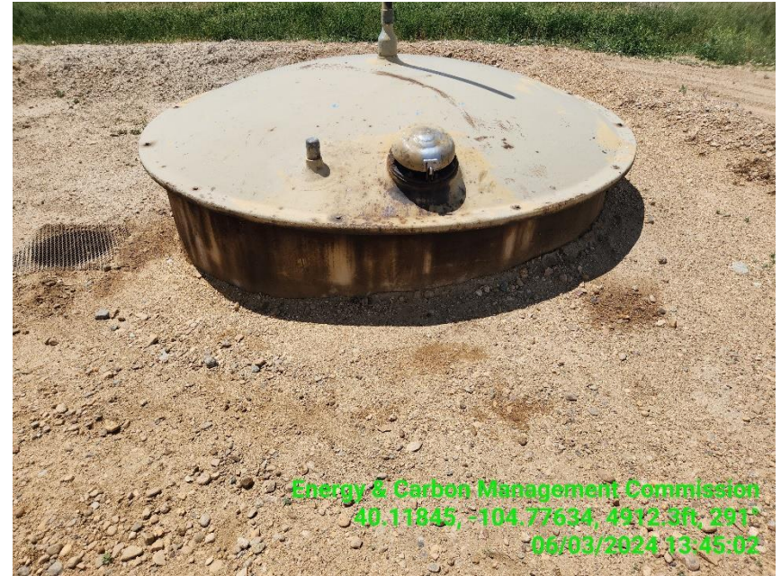
Photo 20 Stained soil around the PW tanks
