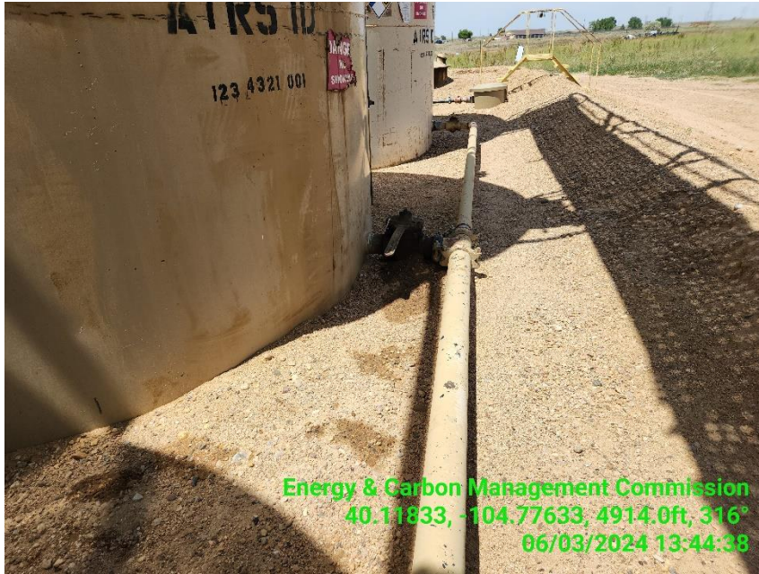
Photo 19 Stained soil by tank load line valve .
