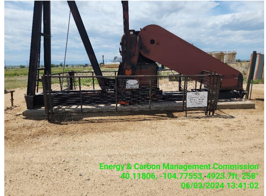
Photo 8 Stained soil around the pump jack base.
