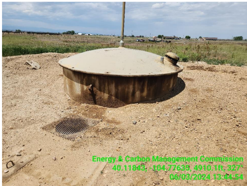
Photo 21 Stained soil by PW tanks.
