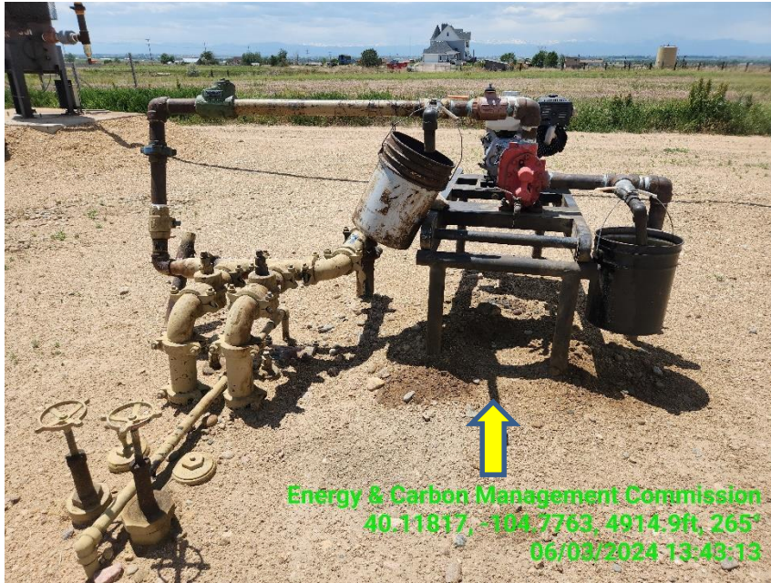
Photo 13 Stained soil by the flow line manifold & aux. pu.mp
