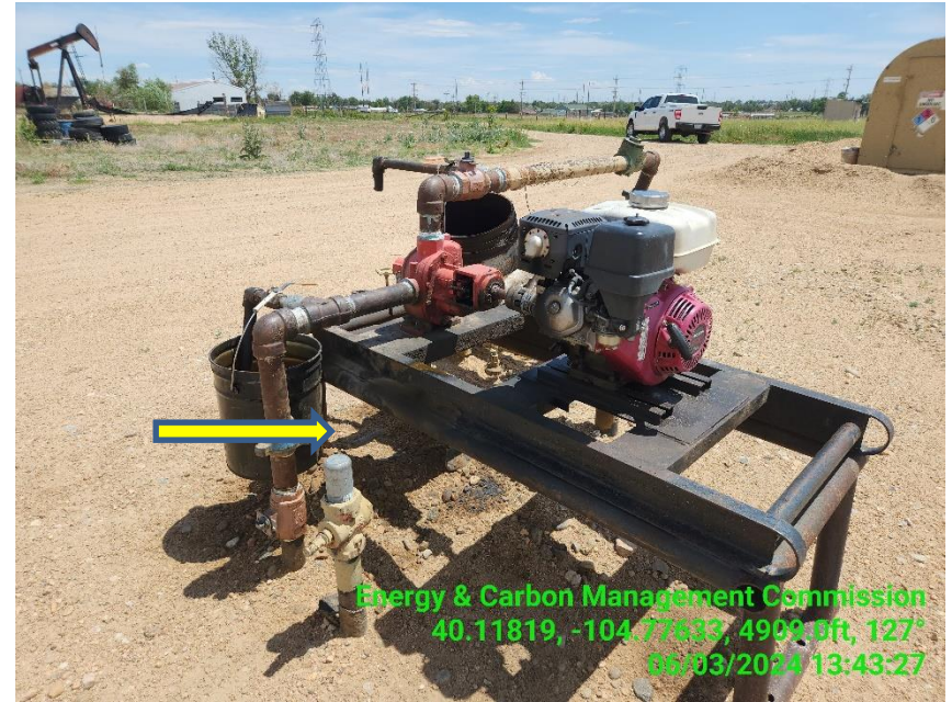
Photo 14 Stained soil by the flow line manifold & aux. pump.
