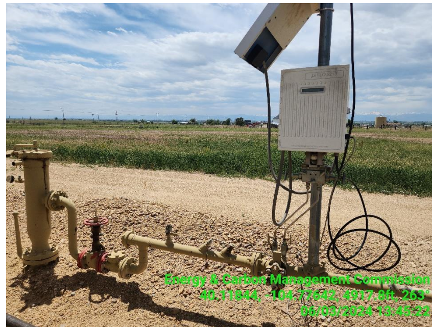
Photo 22 Gas Meter Run.
