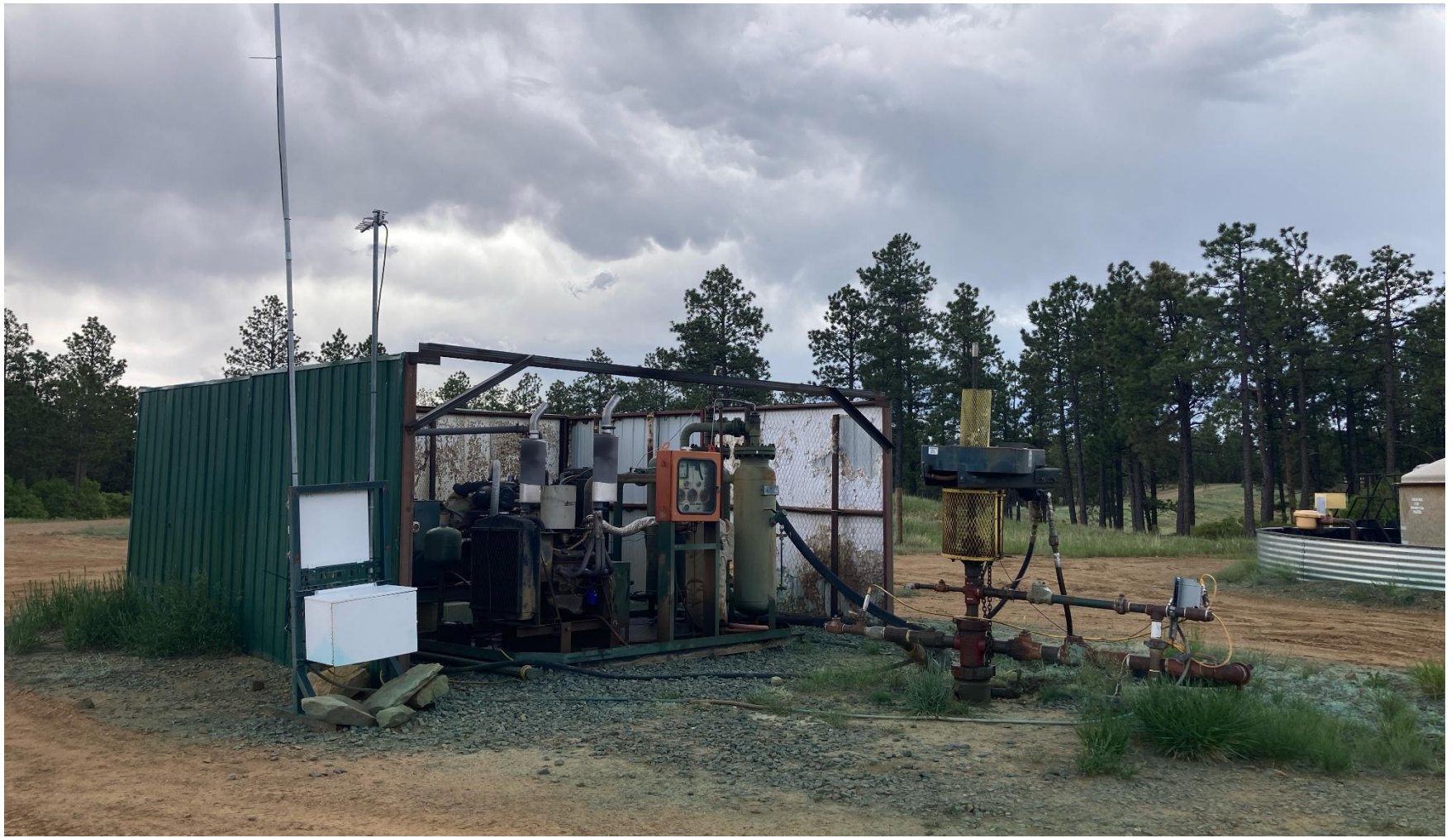
PHOTO 3: WELLHEAD AND EQUIPMENT
