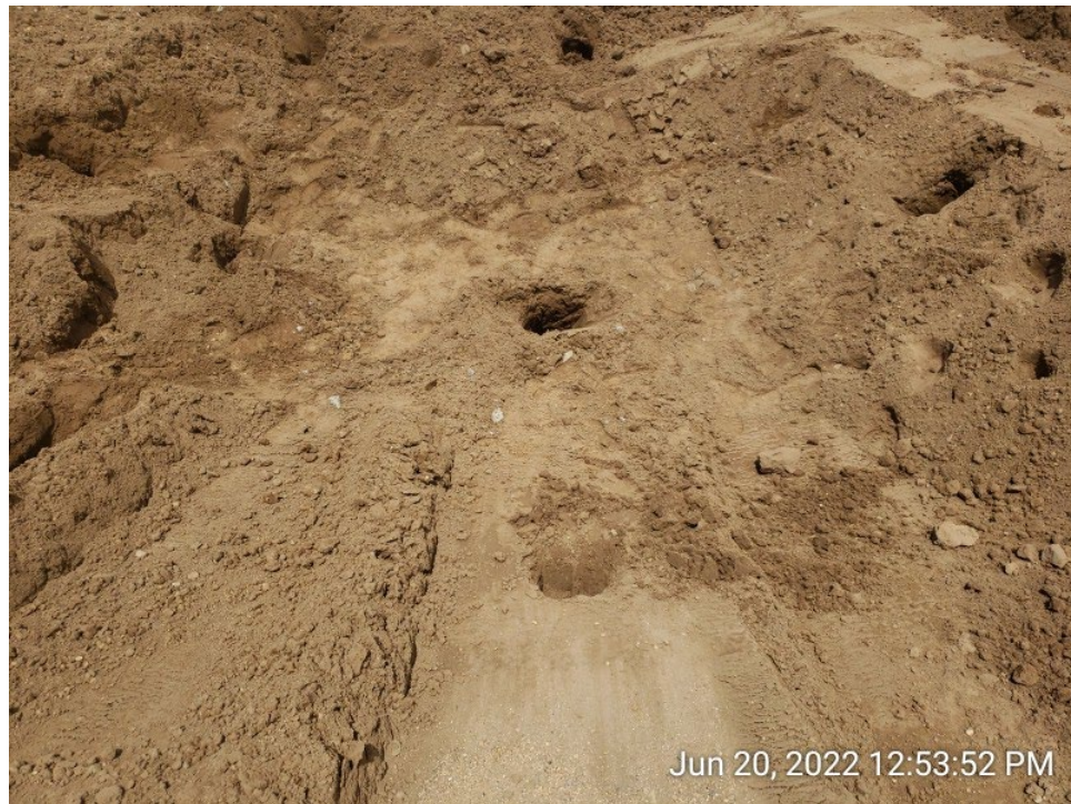
#4A - UPRC-65N64W 23SESW – Base of Eastern Produced Water Vessel Excavation – EPWVB01@7.0' – No Impacts Noted – PID 9.7ppm – Sample Submitted for Lab Analysis – Facing North
