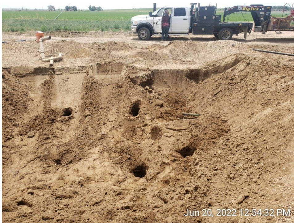
#5C - UPRC-65N64W 23SESW – Southern Sidewall of Western Produced Water Vessel Excavation – WPWVS01@6.0’– No Impacts Noted – PID 0.3ppm – Facing South
