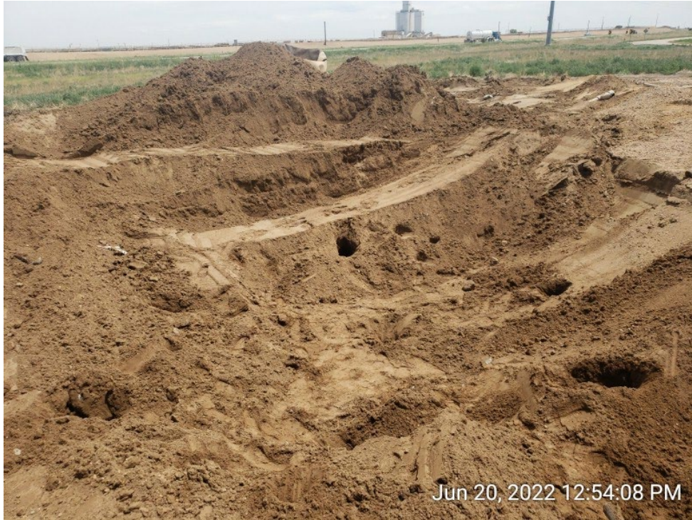
#4D - UPRC-65N64W 23SESW – Eastern Sidewall of Eastern Produced Water Vessel Excavation – EPWVE01@6.0' – No Impacts Noted – PID 0.8ppm – Facing East
