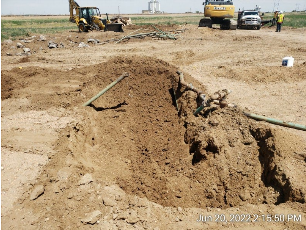
#6B - UPRC-65N64W 23SESW – ASTs and PWVs Dumplines – Separator Tie-In – DL01@3.0' – No Impacts Noted – PID 1.0ppm – Facing East
