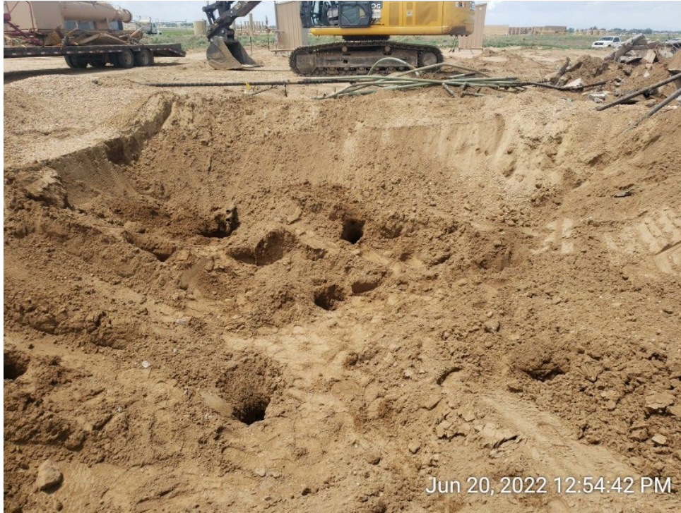
#5D - UPRC-65N64W 23SESW – Western Sidewall of Western Produced Water Vessel Excavation – WPWVW01@6.0’– No Impacts Noted – PID 1.7ppm – Facing West
