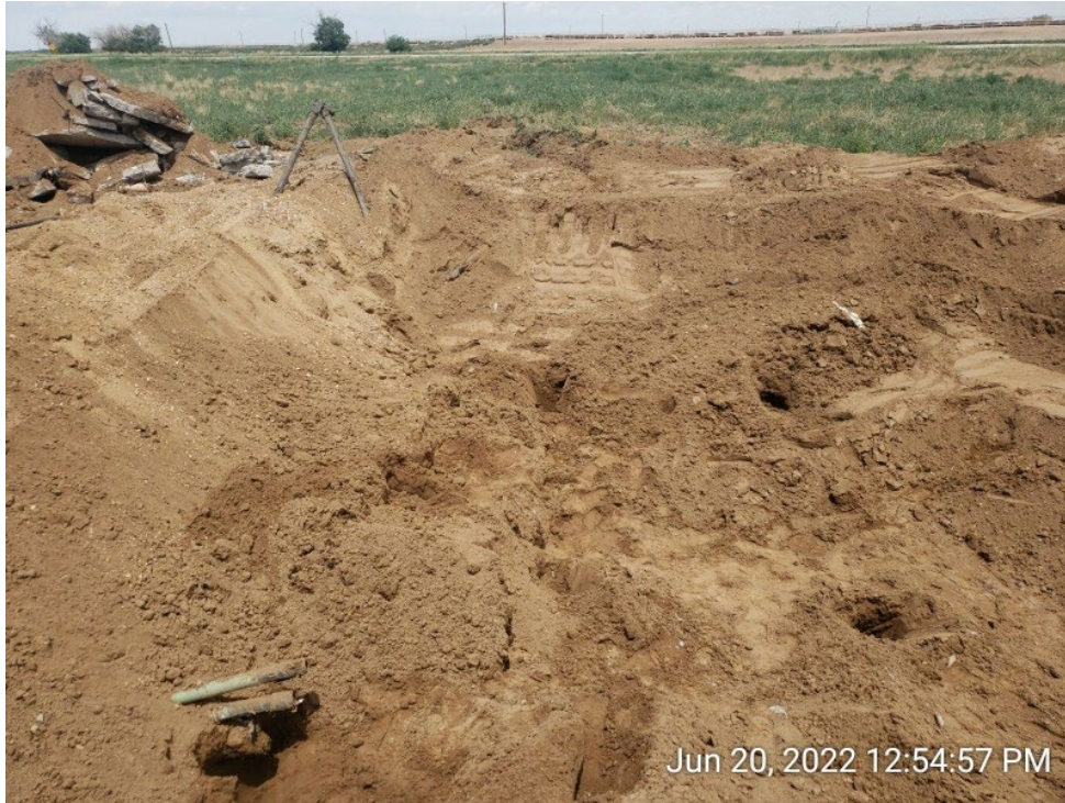
#5B - UPRC-65N64W 23SESW – Northern Sidewall of Western Produced Water Vessel Excavation – WPWVN01@6.0’– No Impacts Noted – PID 5.4ppm – Sample Submitted for Lab Analysis – Facing North
