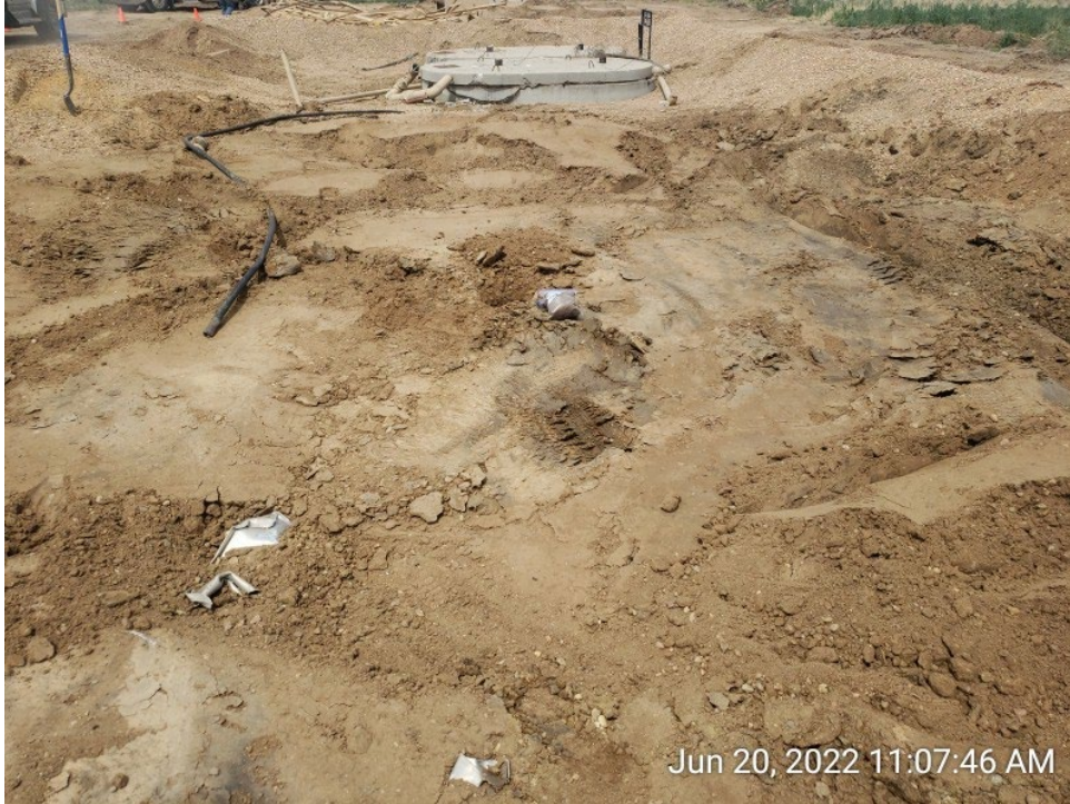
#1A - UPRC-65N64W 23SESW – Eastern Above Ground Storage Tank – EAST01@6.0” – No Impacts Noted – PID 0.3ppm – Sample Submitted for Lab Analysis – Facing West
