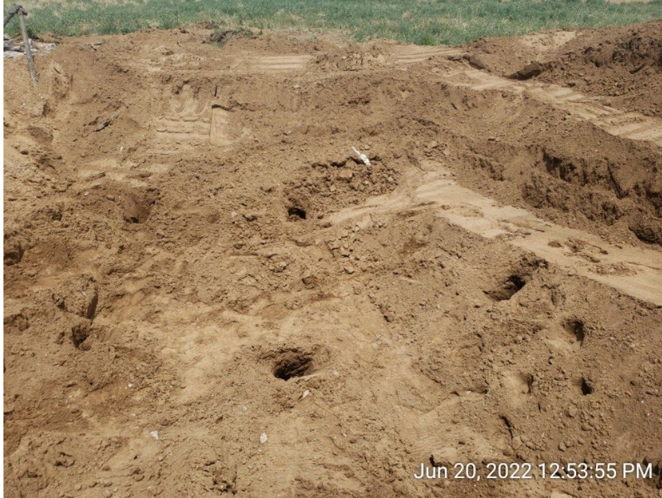
#4B - UPRC-65N64W 23SESW – Northern Sidewall of Eastern Produced Water Vessel Excavation – EPWVN01@6.0’ – No Impacts Noted – PID 1.0ppm – Sample Submitted for Lab Analysis – Facing North
