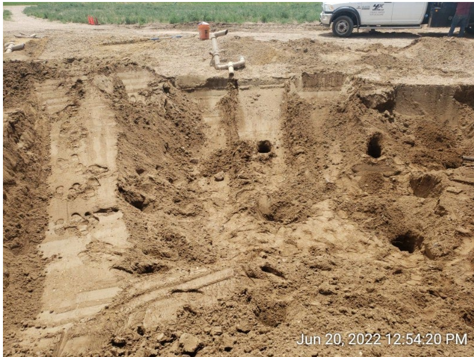
#4C - UPRC-65N64W 23SESW – Southern Sidewall of Eastern Produced Water Vessel Excavation – EPWVS01@6.0’ – No Impacts Noted – PID 0.6ppm – Facing South
