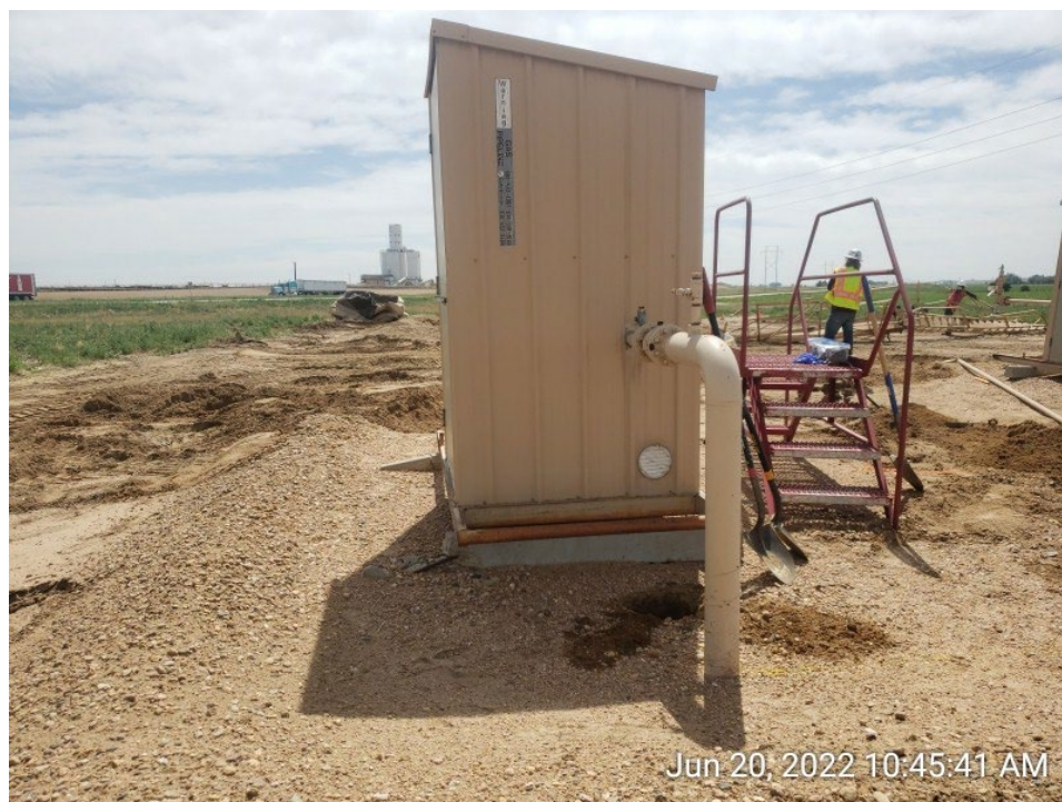
#10A - UPRC-65N64W 23SESW – Northern Third-Party Meter Shed – MET01@6.0” – No Impacts Noted – PID 1.3ppm – Facing East
