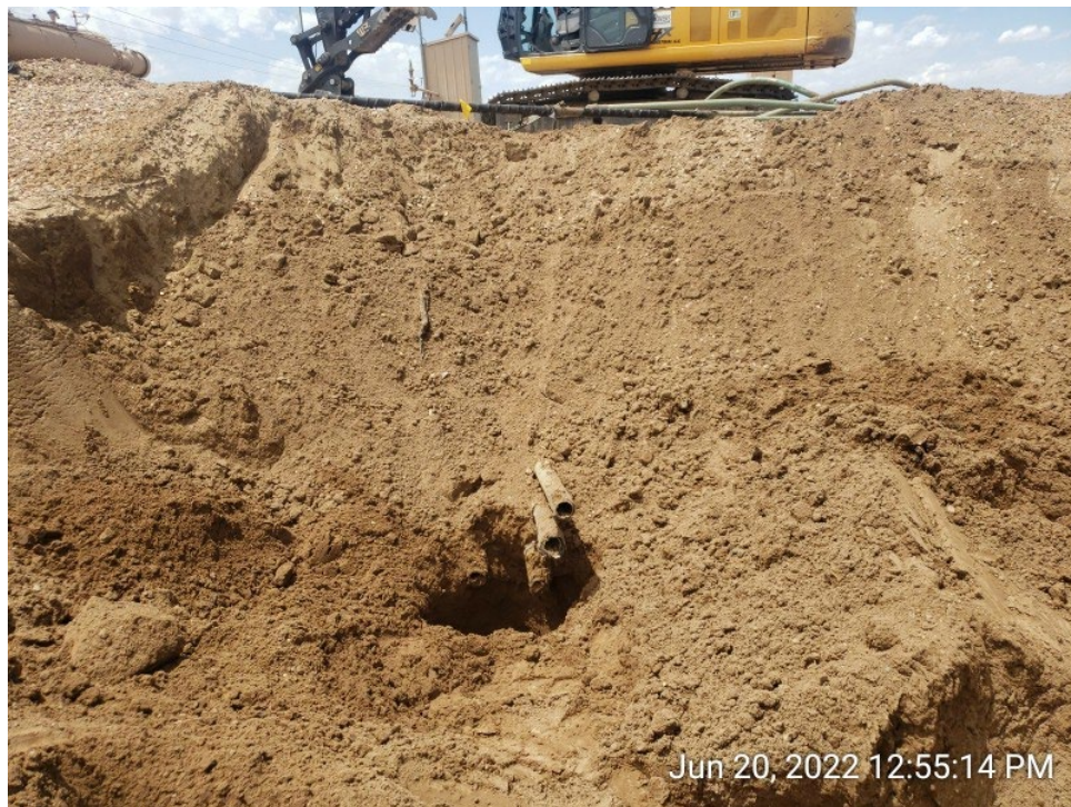
#6A - UPRC-65N64W 23SESW – ASTs and PWVs Dumplines – Southwest Corner of PWVs Excavation – DL02@6.0’– No Impacts Noted – PID 0.6ppm – Facing West
