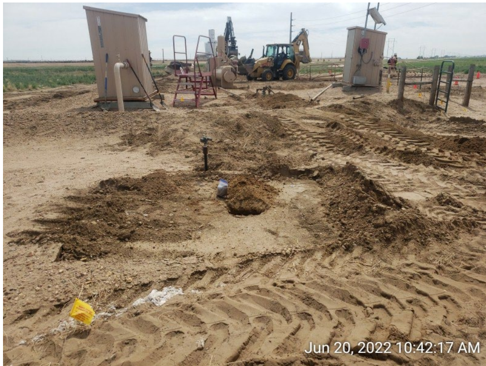
#9A - UPRC-65N64W 23SESW – Southern Combustion Unit – ECD02@6.0” – No Impacts Noted – PID 2.1ppm – Facing East
