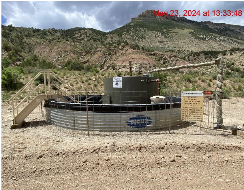
Tank Battery – Photo #01372
