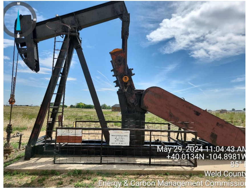
Photo 2 well head and equipment
