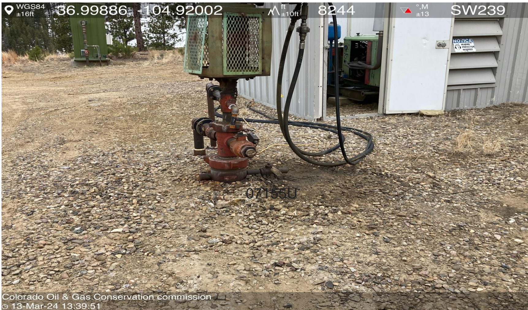
PHOTO 4: IMPACTED SOIL AROUND WELLHEAD.
