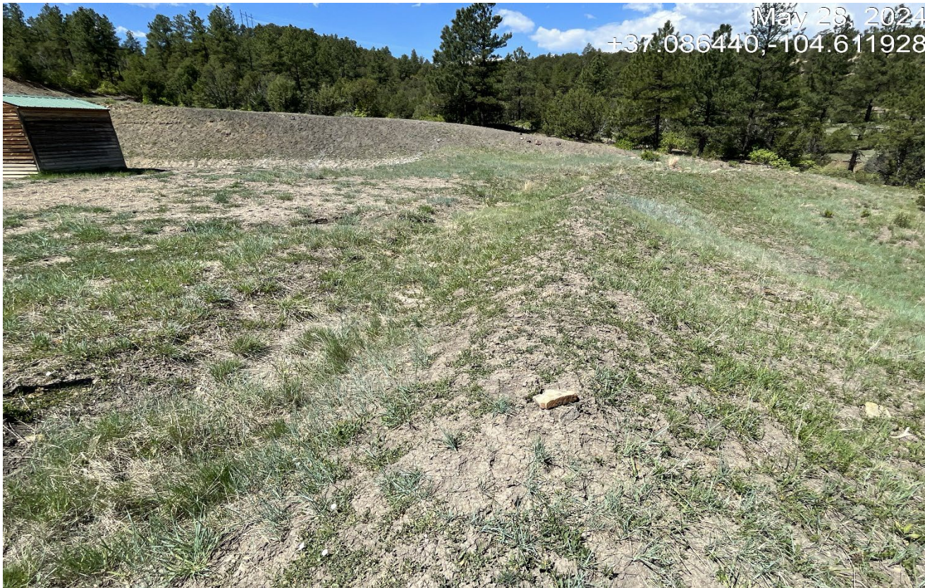
Photo 2. The perennial vegetation is established along the fill slope.
