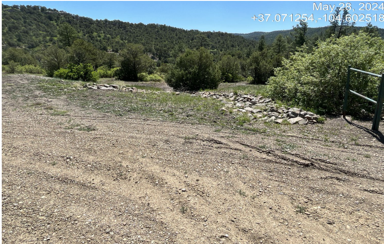
Photo 3. There is rip/rap outlet protection along the south side of the location.
