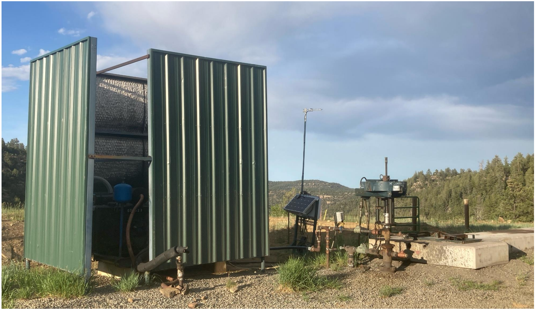
PHOTO 3: R WELLHEAD AND EQUIPMENT
