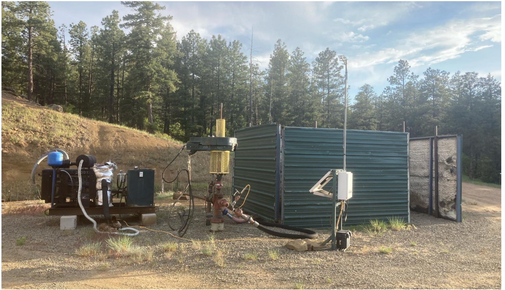
PHOTO 4: V WELLHEAD AND EQUIPMENT
