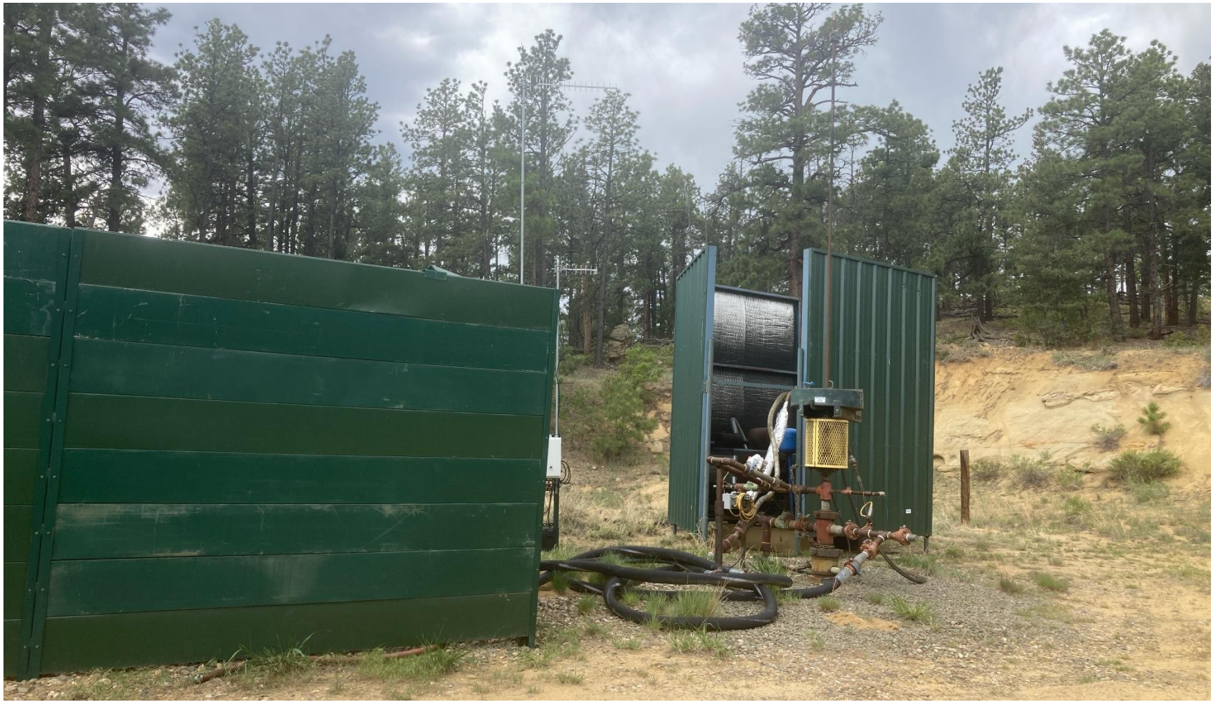
PHOTO 4: R WELLHEAD AND EQUIPMENT
