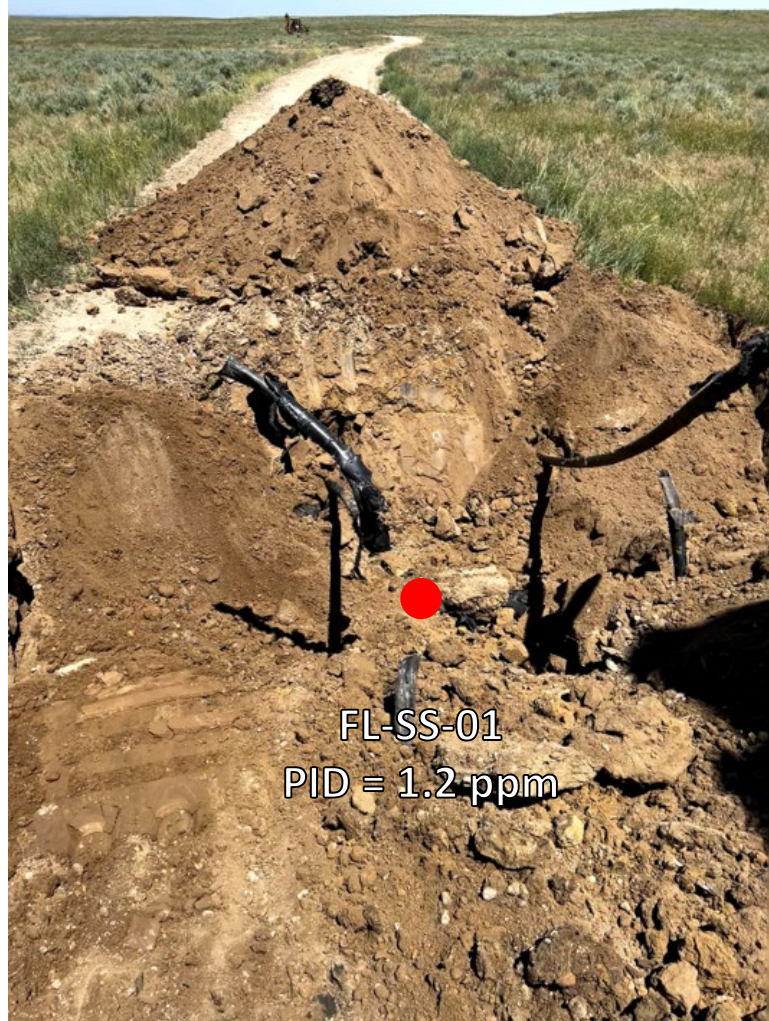
Looking north at flowline directional change
