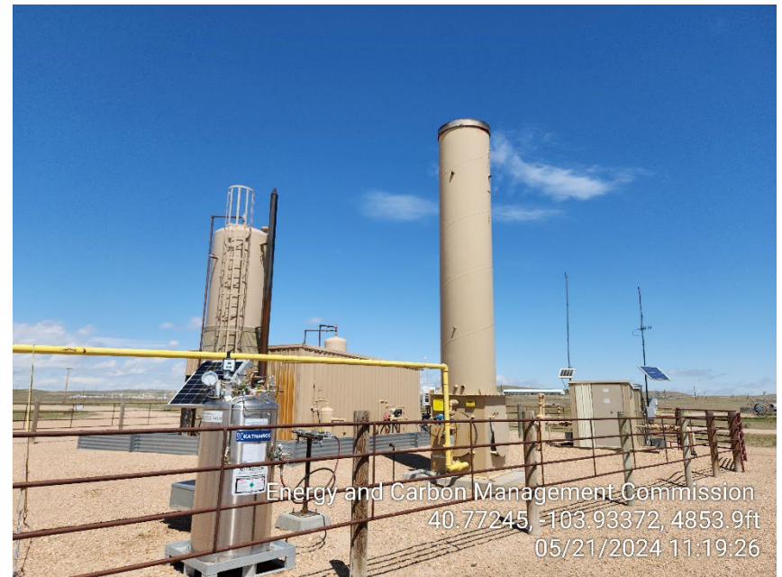
Photo 8 – ECD and Nitrogen Tank
