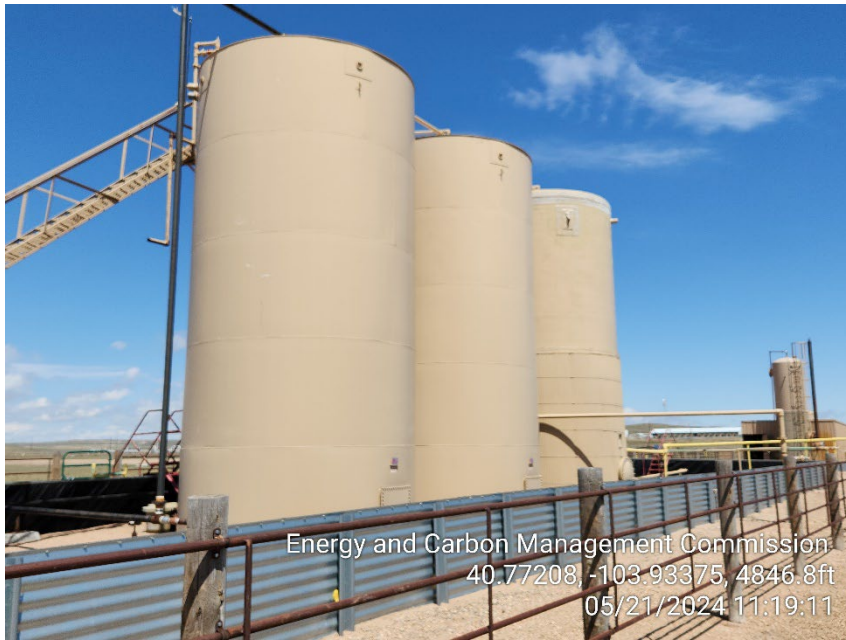
Photo 7 – Tank Battery – Backside of Tanks
