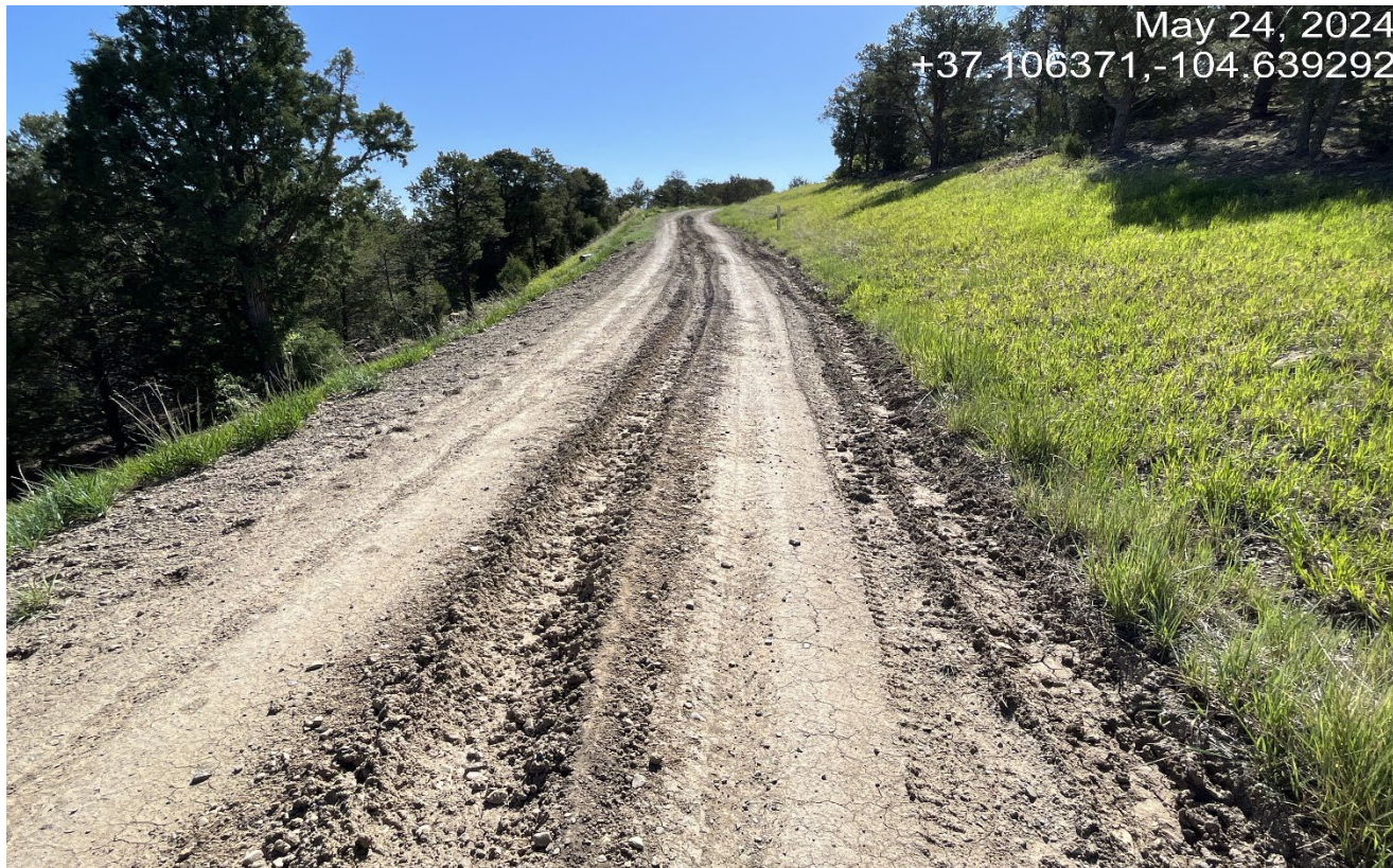
Photo 1. Facing southeast along the access road. There is vehicle rutting along the road that will need to be repaired.
