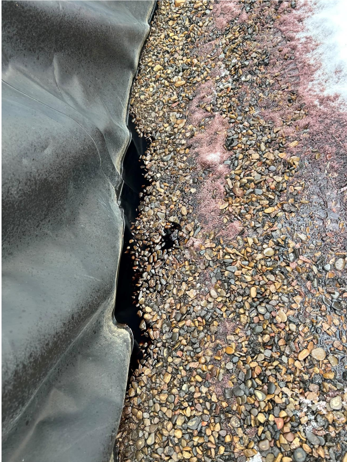
12/10/23 – Photo showing integrity of lined containment following release
