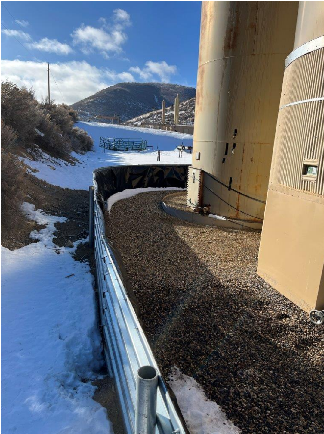
12/14/2023 – Photo showing containment following free liquid removal
