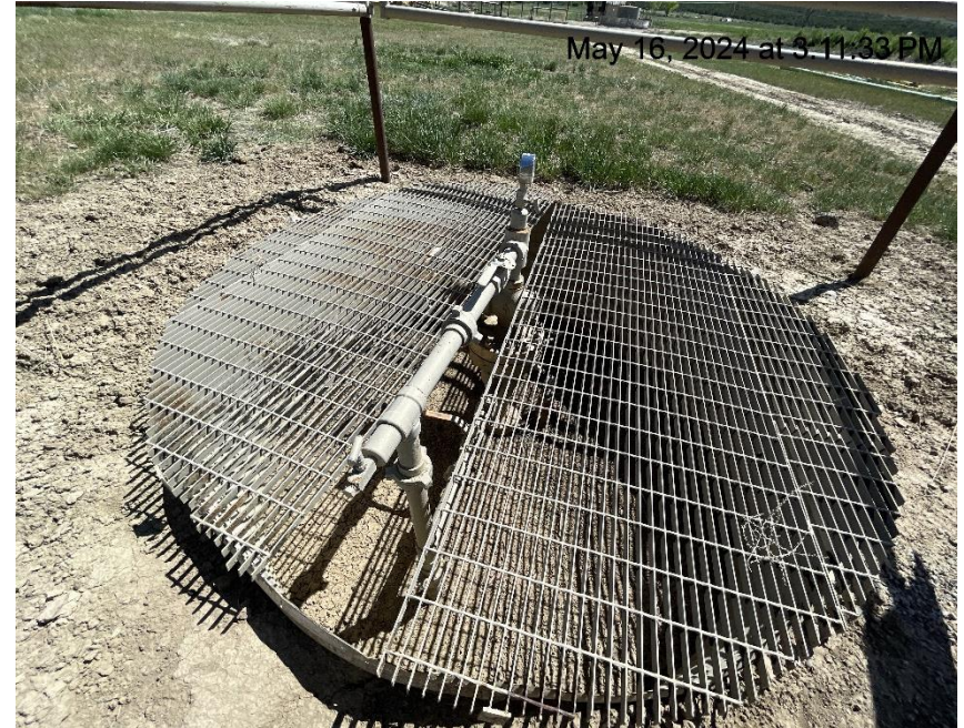
Photo # 7533 Cellar lacks wildlife egress - Please refer to inspection 708903824 for corrective action
