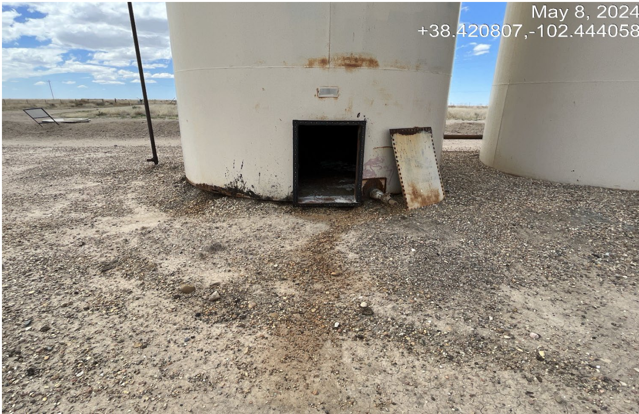
Photo 3. There is an open hatch on the backside of the tank. This needs to be covered to prevent wildlife entry.
