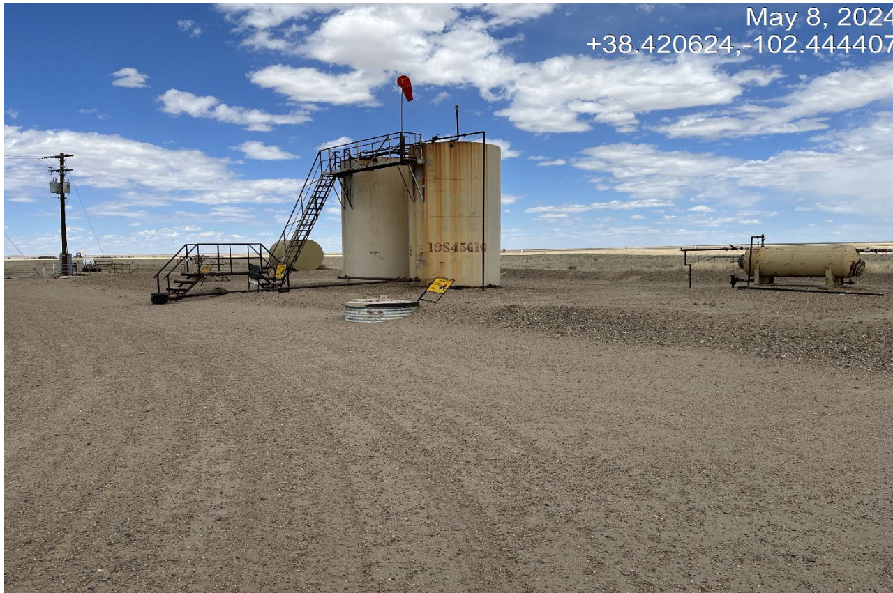
Photo 2. Facing northeast towards the tank battery. The wind sock has been replaced.
