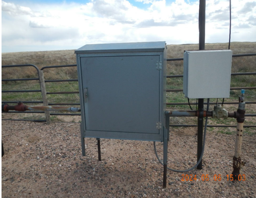
3. Flowline mounted gas meter box.
