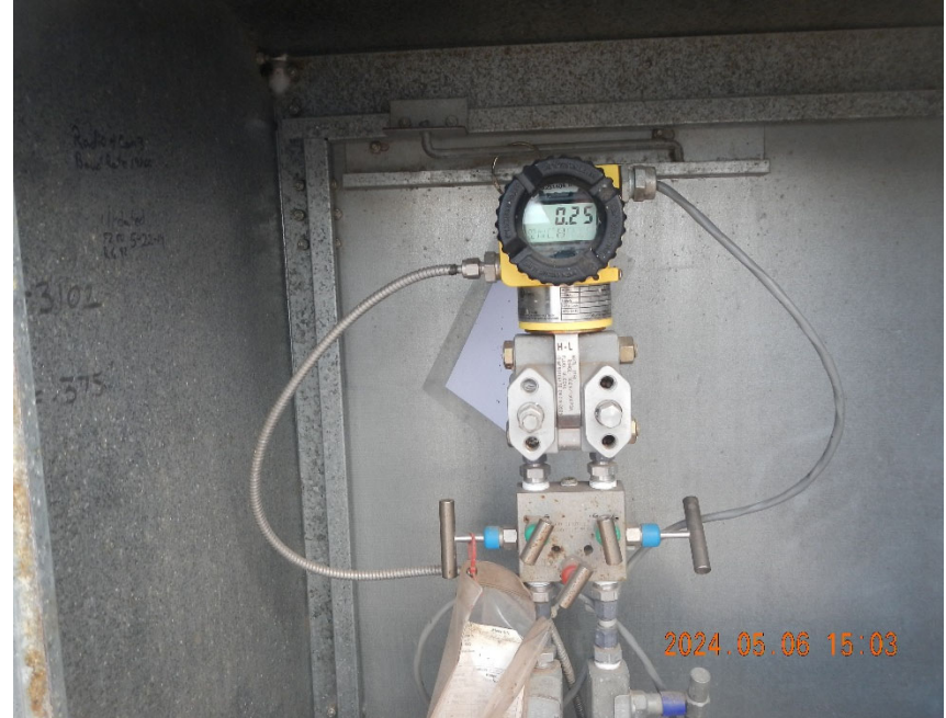
4. Digital gas meter inside meter box.
