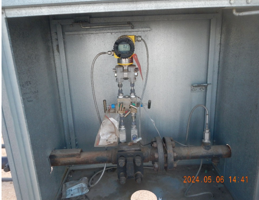
3. Digital gas meter inside meter box.
