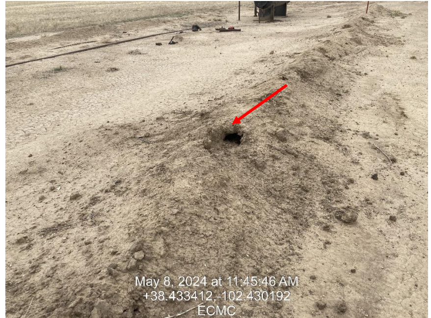
Photo 10 – Hole in berm
