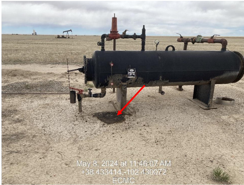
Photo 9 – Impacted soils at Heater Treater
