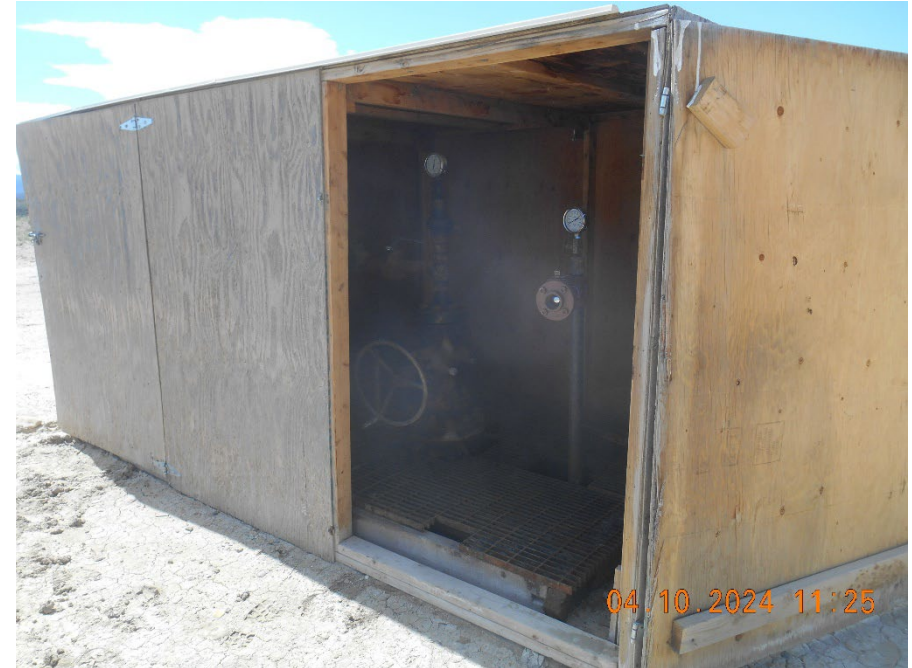
Injection Wellhead inside housing
