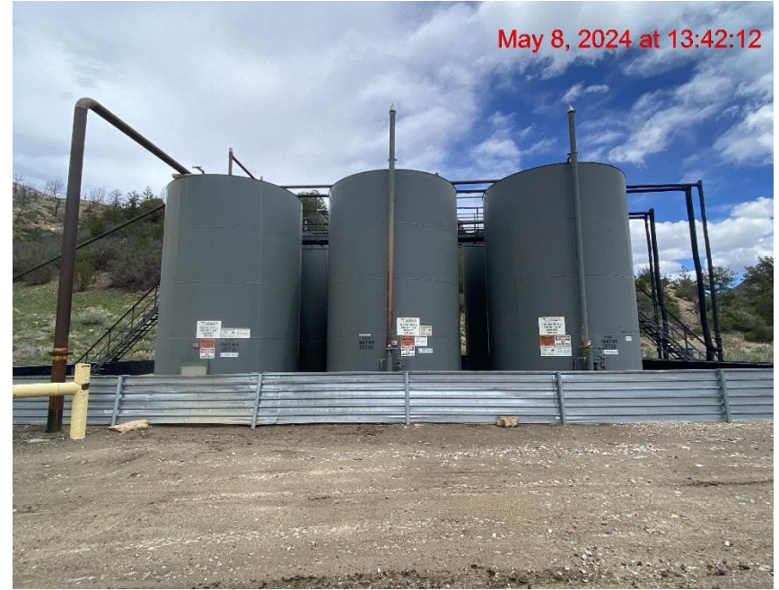
Tank Battery – Photo #01019
