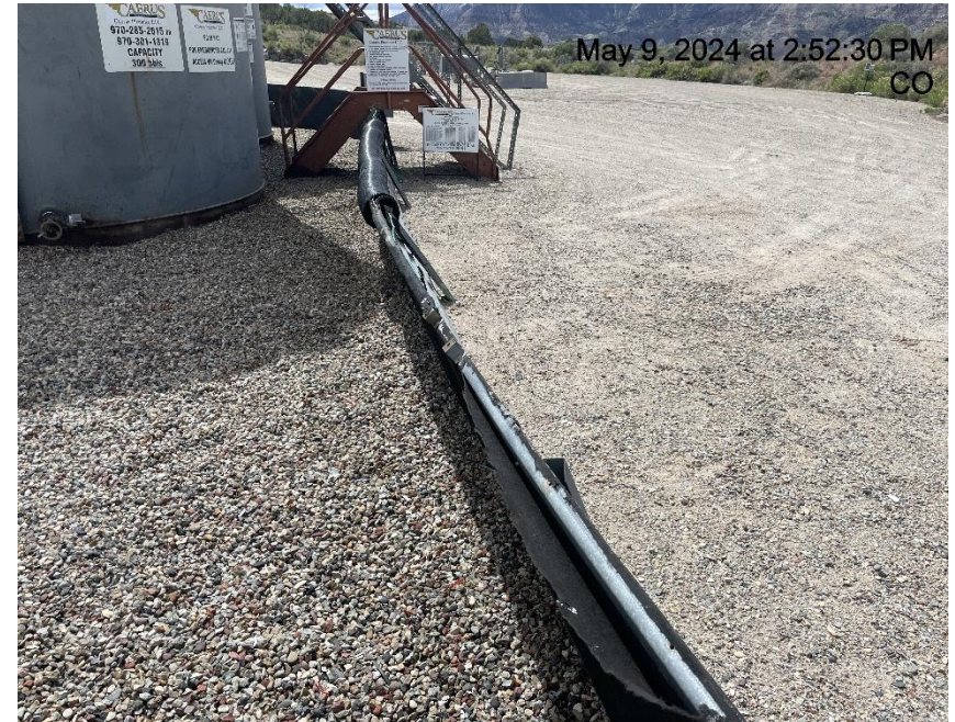
Photo # 6539 Tank containment damaged/buckling
