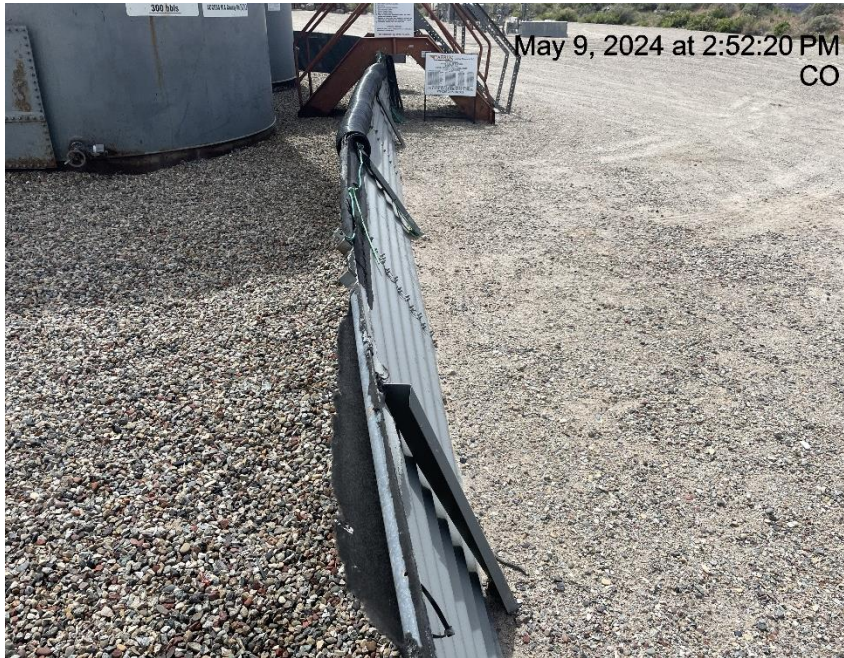
Photo # 6538 Tank containment damaged/buckling
