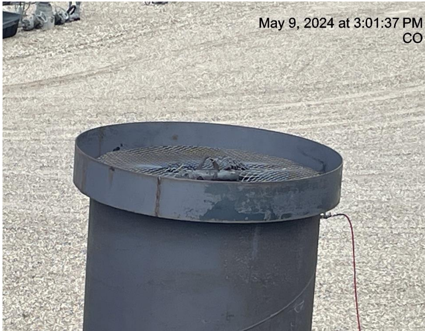
Photo # 6536 Bird protection on ECD damaged & needs maintenance/wildlife hazard/available for entry by wildlife
